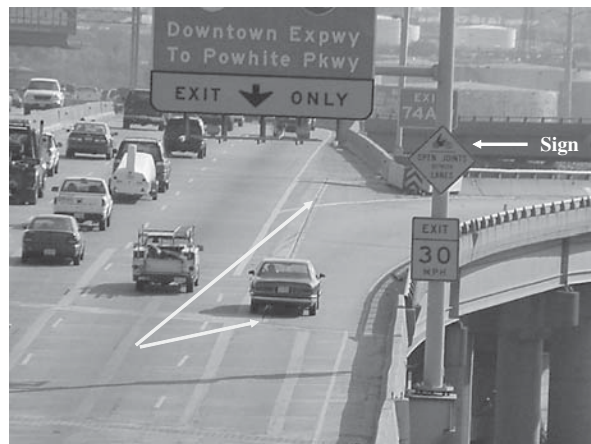
EXHIBIT V-23 Irregular Roadway Surface and Advance Warning Sign
