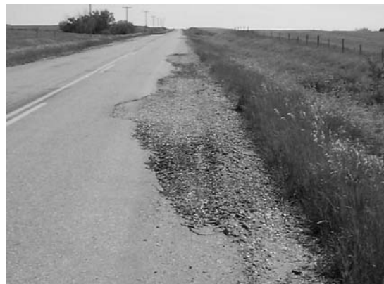
EXHIBIT V-10 Deteriorating Pavement and Gravel from Poor Roadway Maintenance
