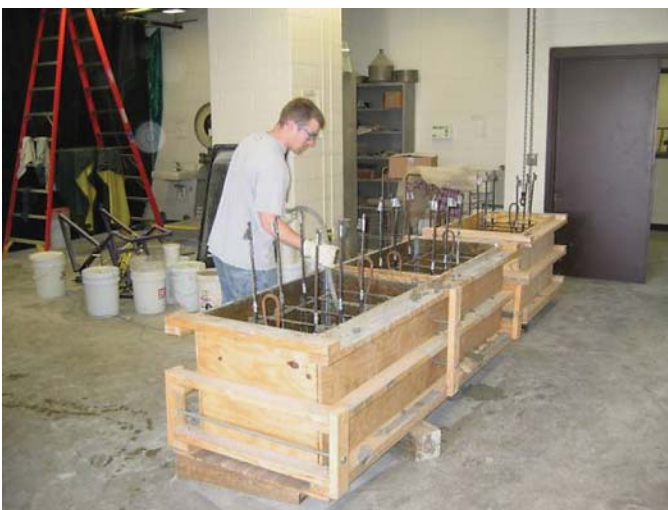
Figure B-22. View of large block forms during concrete pour. The student is internally vibrating the concrete.
