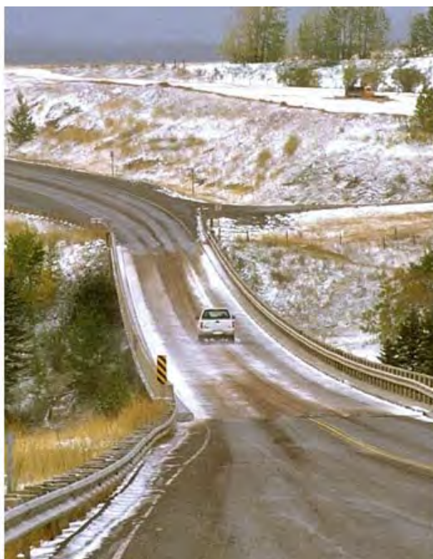
FIGURE 4 Ice remains on a bridge deck while approach roads are clear.
