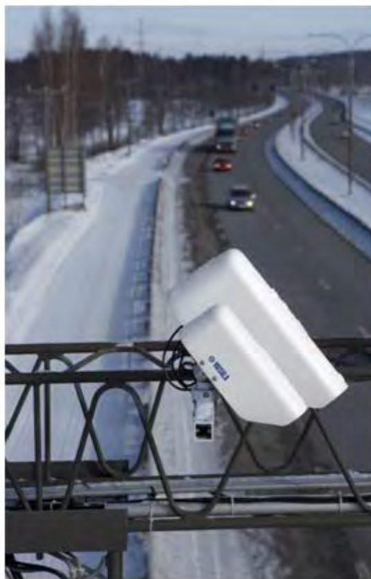
FIGURE 2 Nonintrusive sensors mounted on an overhead gantry.
