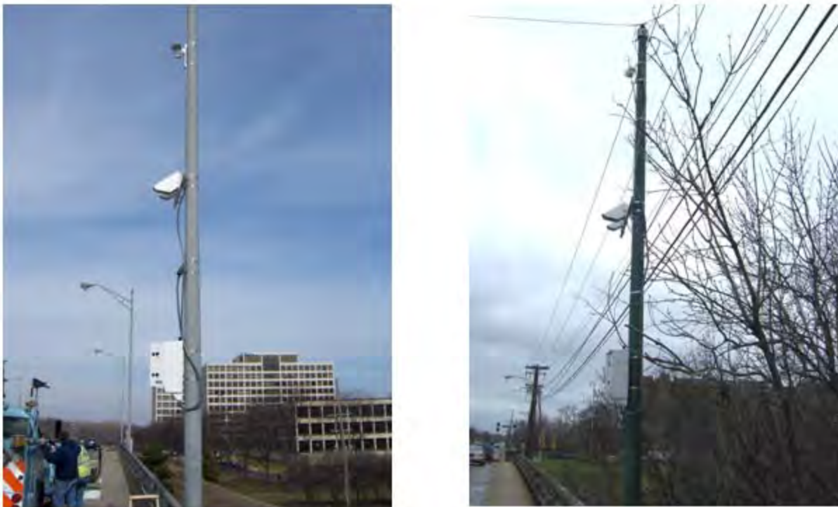
FIGURE 5 Nonintrusive sensors mounted on existing street furniture in Chicago.
