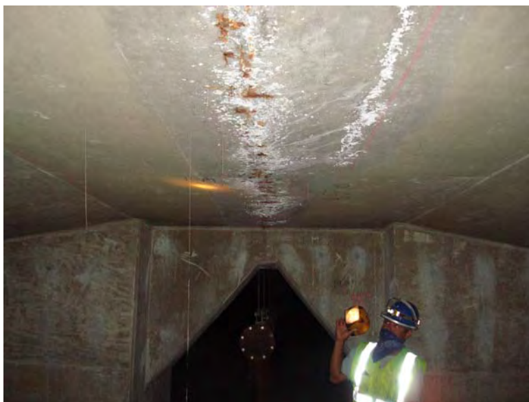
FIGURE 2 Presence of efflorescence, delamination, and spall observed on post-tensioned box girders.
