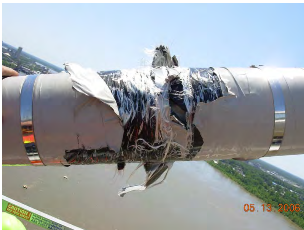
FIGURE 8 Separation of PE transverse joints.
