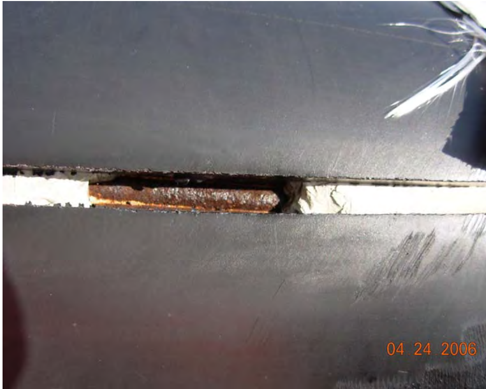
FIGURE 5 PE pipe split; UV protection tape missing.
