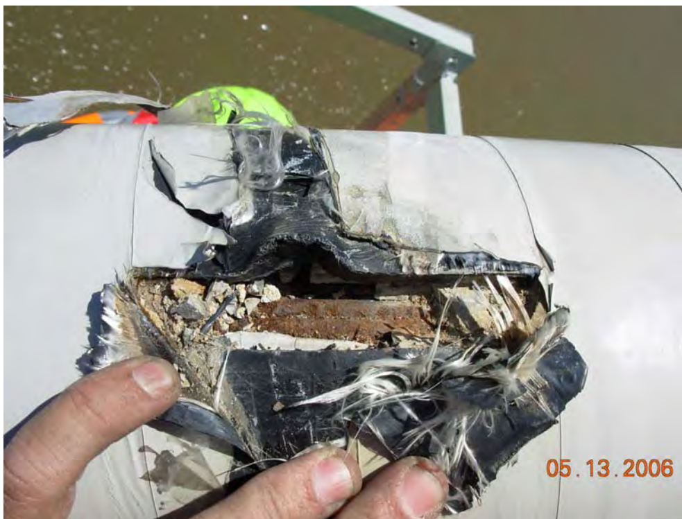
FIGURE 7 PE sheathing split, wire corroded, and wire not providing protection.
