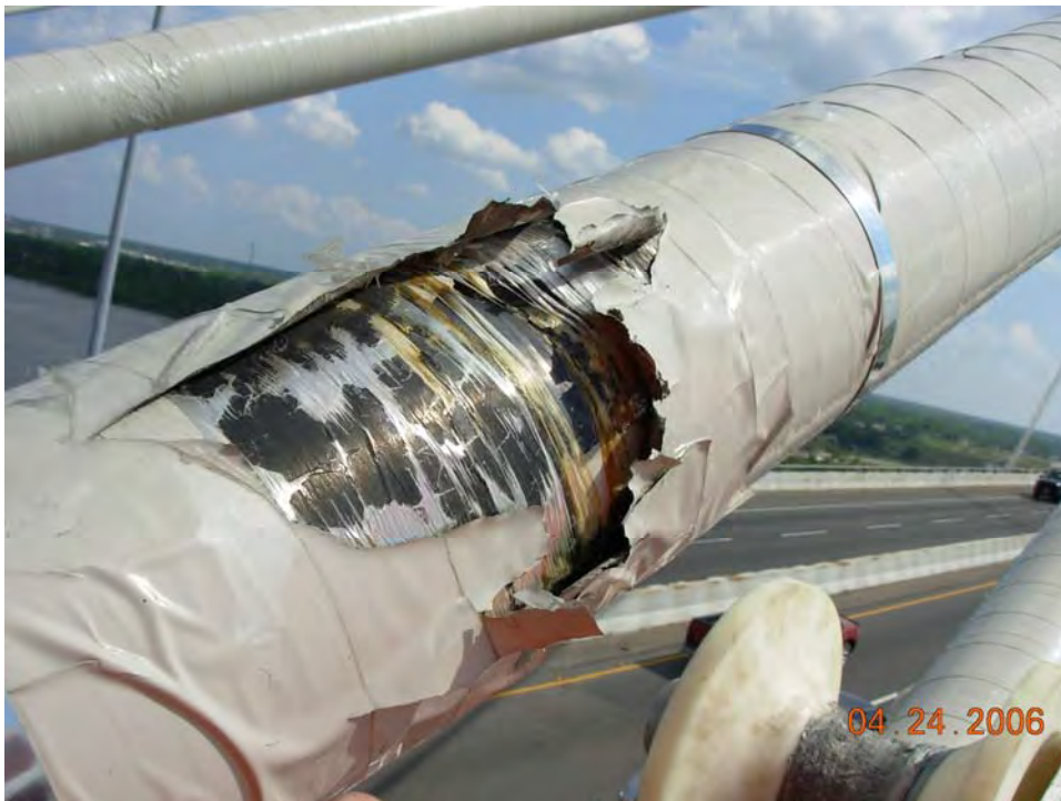
FIGURE 6 Burst and damaged protective tape.
