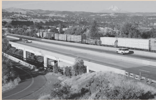
On I-84, the major highway that runs through the Columbia River Gorge National Scenic Area, 17 bridges are slated for repair or replacement.
