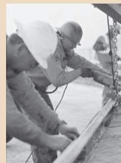
Workers install a guardrail along US-97 during the first stage of the Oregon bridge program.
