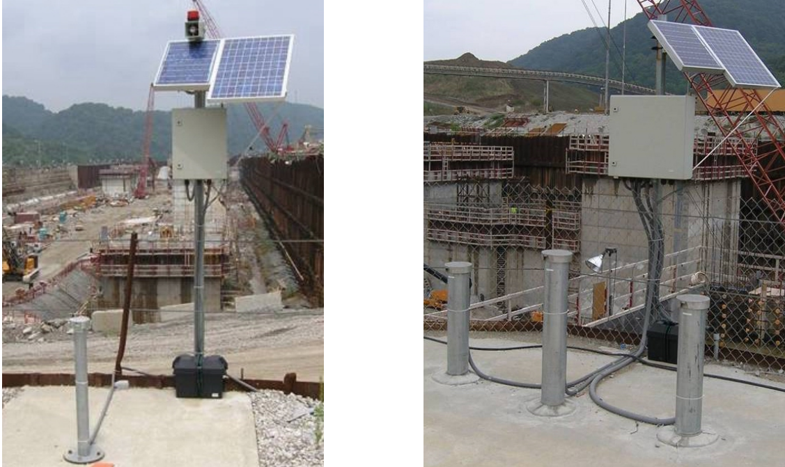
FIGURE 20 ADAS with solar power and communication system (Myers et al., 2000).
