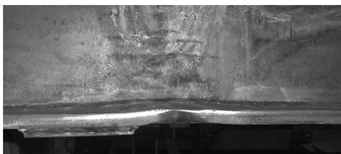
Figure 2.50. Residual damage on Specimen 1D/R-2.
