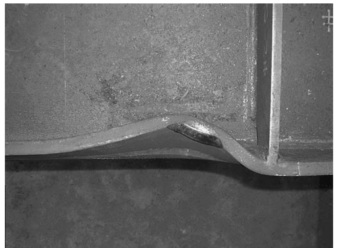
Figure 1.11. Typical local damage from the drop-weight machine impact.
