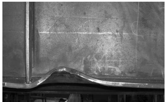
Figure 2.27. Localized damage at a transverse stiffener detail.
