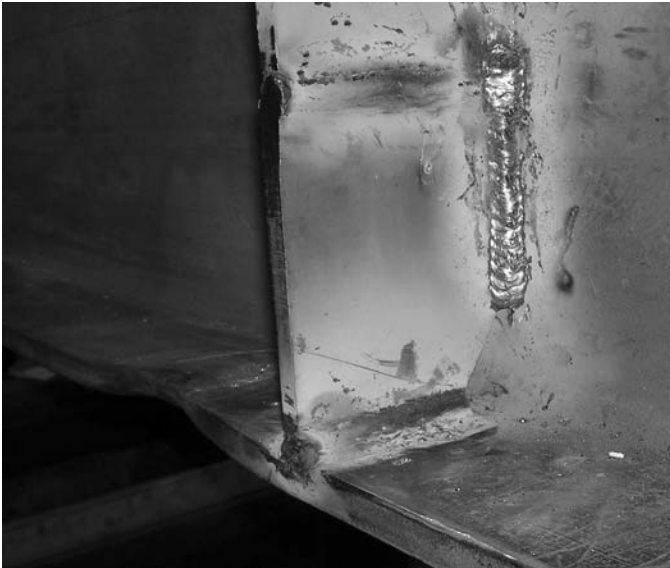
Figure 2.24. Portion of stiffener replaced using a welded repair following the heat-straightening repair.
