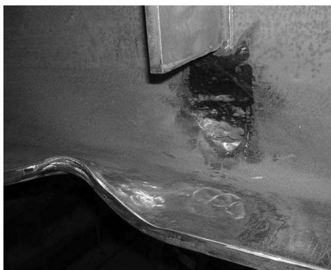
Figure 2.22. Portion of stiffener removed prior to heat-straightening repair.
