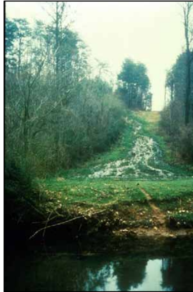
FIGURE 3-31 Sewage from clogged system overflowing into storm drainage system. SOURCE: Robert Pitt, University of Alabama.
