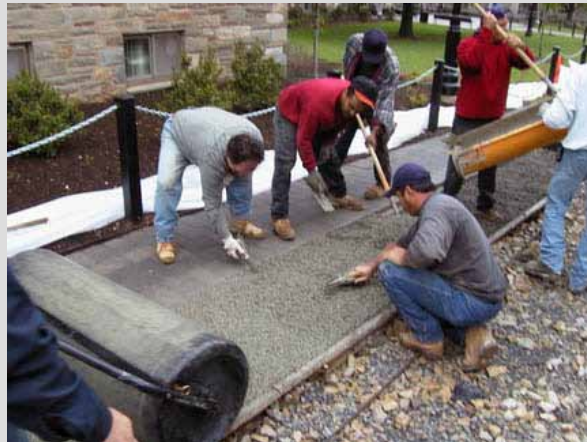
FIGURE 5-34 Infiltration bed under construction. Pervious concrete has functionality and workability similar to that of regular concrete. However, the pervious concrete mix lacks the sand and other fine particles found in regular concrete. This creates a significant amount of void space which allows water to flow relatively unobstructed through the concrete. This site was the first attempt at creating a pervious concrete SCM in the area, and there were construction and material problems. Since that time the industry has matured, and a second site on campus constructed in 2007 has not had any significant difficulties. SOURCE: Reprinted, with permission, from VUSP. Copyright by VUSP.
