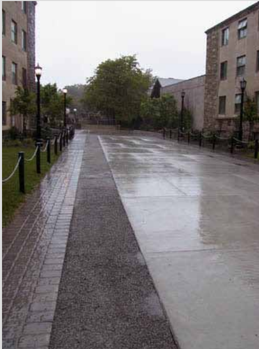
Note the runoff from impervious concrete spilling over to the pervious concrete. SOURCE: Robert Traver, Villanova University
