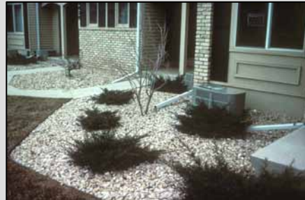
A disconnected roof drain (drains to pervious area)
