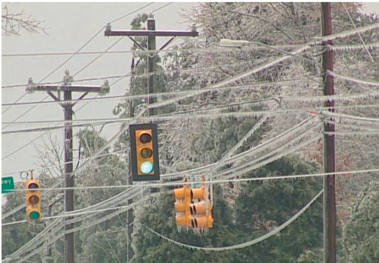
December 2002 ice storm in the Western Carolinas. SOURCE: Nick Keener, Duke Energy.
