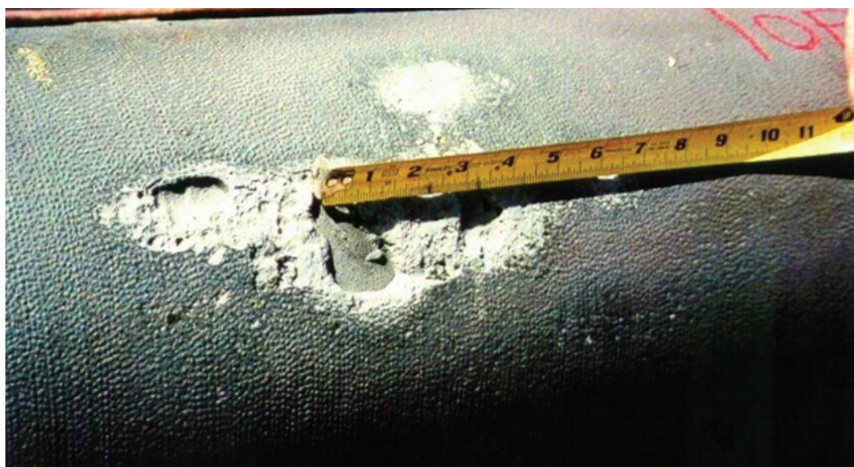
FIGURE 3-5 In Colorado Springs, Colorado, force main corrosion where only polyethylene lining was holding sewage pressure. SOURCE: Courtesy of William Spickelmire, RUSTNOT Corrosion Control Services, Inc.
