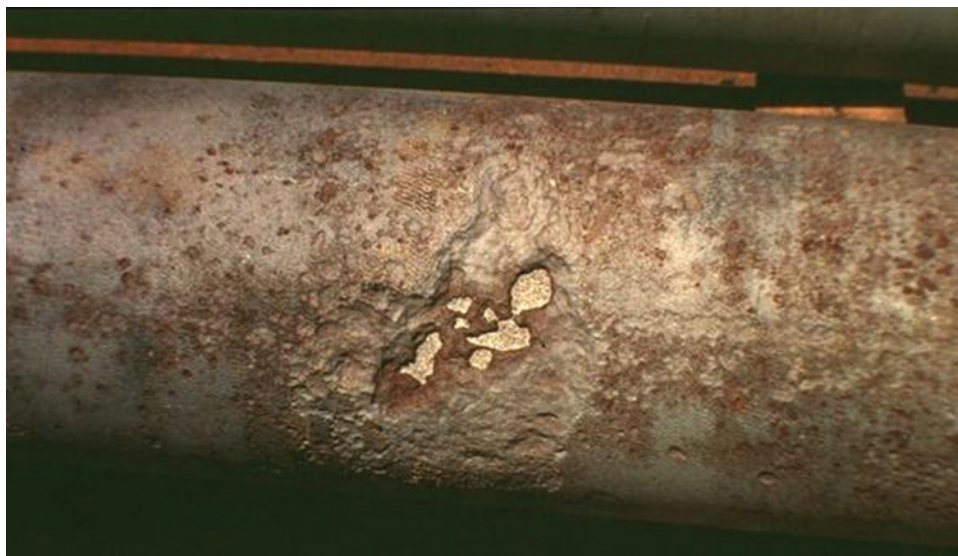
FIGURE 3-2 In Vancouver, British Columbia, ductile iron pipe with polyethylene encasement after sandblasting where graphitic corrosion and cement mortar lining previously held 650 pounds per square inch water pressure. SOURCE: Courtesy of William Spickelmire, RUSTNOT Corrosion Control Services, Inc.
