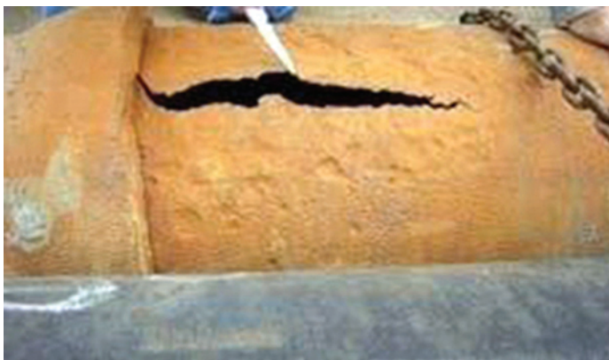
FIGURE 3-7 Location of 2004 leak on 16-inch Class 250 (300 mil thick) ductile iron pipe with polyethylene encasement and cathodic protection in North Dakota. SOURCE: Courtesy of Joe Bichler, Bartlett and West Engineers.
