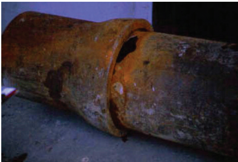
FIGURE 3-9 In California City, California, major corrosion damage on ductile iron pipe with polyethylene encasement and cathodic protection with joint bond on opposite side of pipe. SOURCE: Courtesy of William Spickelmire, RUSTNOT Corrosion Control Services, Inc.
