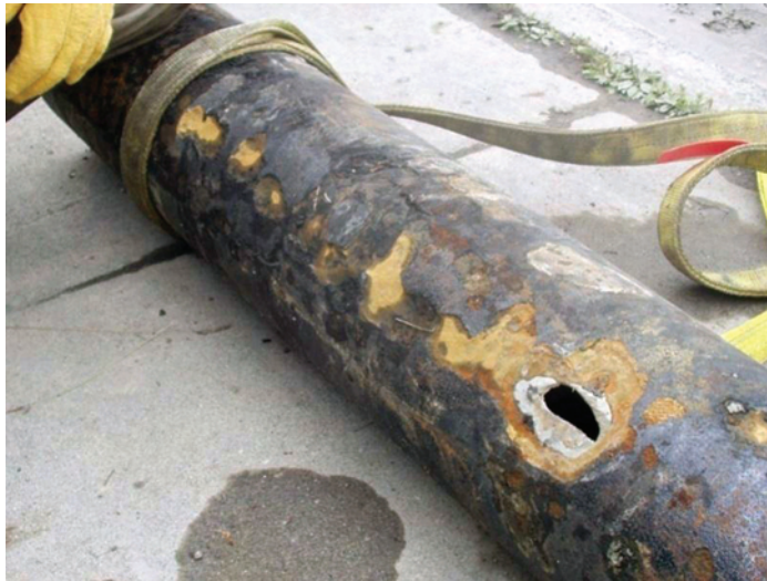
FIGURE 3-4 Nine-year-old 8-inch ductile iron pipe with polyethylene encasement in Anchorage, Alaska. SOURCE: Mark Corsentino, Presentation entitled “Corrosion and Mitigation of AWWU Infrastructure,” given at the Alaska Water and Wastewater Management Association 48th Annual Statewide Conference: Anchorage, Alaska, May 2008.
