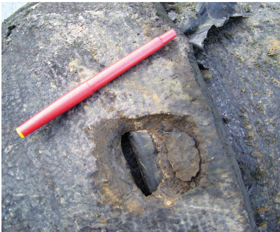
FIGURE 3-8 Location of leak on bottom of cathodically protected 16-inch ductile iron pipe with polyethylene encasement in Ohio. SOURCE: Courtesy of Gregg Loesch, Akron Public Utilities Bureau.
