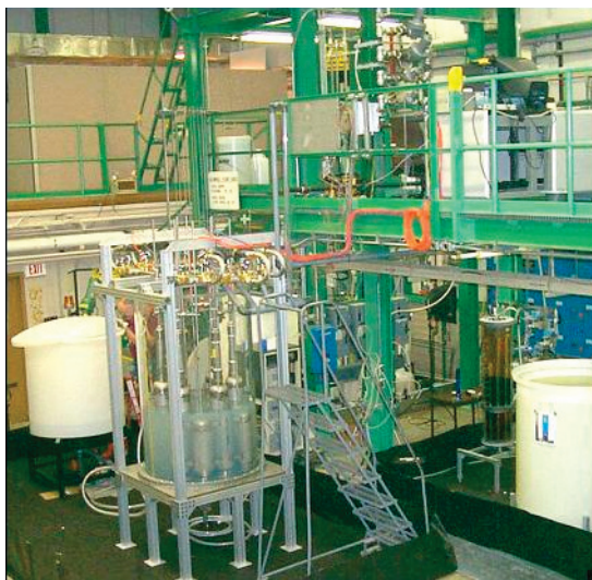
FIGURE 3.3 High-bay building for engineering tests. High-bay buildings provide two or more stories of vertical space for testing or demonstration of large equipment, which is typically required for waste processing. In this photo, pulse jet mixers are being tested for use in Hanford's Waste Treatment Plant. Thorough testing of such newly designed equipment is necessary because it must operate reliably as designed, and with little or no opportunity for maintenance, once placed into radioactive service.
