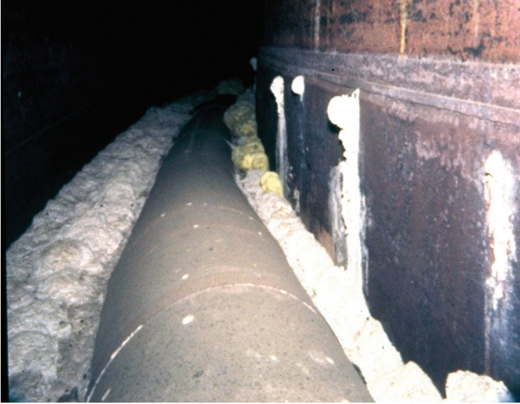
FIGURE 2.4 Salt accumulated in a tank annulus. Double-walled tank construction helped to prevent the release of radioactive waste into the environment. In this figure minor leaks from the primary wall (right) have accumulated in the annulus. SRNL recently developed a robotic crawler for cleaning the tank wall. SOURCE: Department of Energy.
