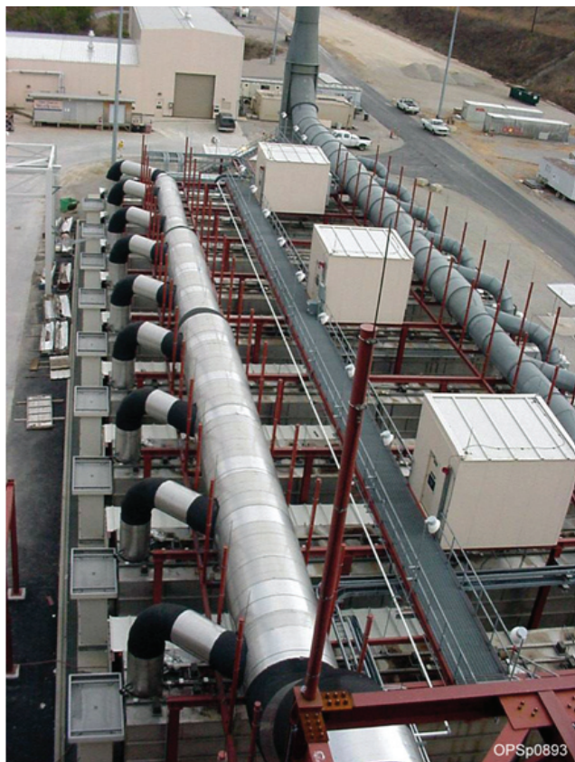
FIGURE 2-1 The nine activated carbon filter units for the MDB HVAC system. SOURCE: Robie Jackson, Waste Management Manager, ANCDF, and Tracy Smith, Trial Burn Manager, ANCDF, “The use of carbon at ANCDF,” Presentation to the committee, June 5, 2008.
