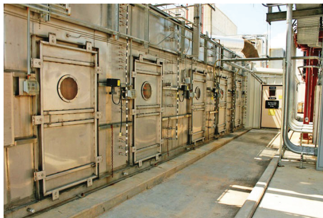
FIGURE 2-10 Vestibule on the side of an MDB HVAC unit. SOURCE: Photograph taken at ANCDF and provided courtesy of ANCDF.
