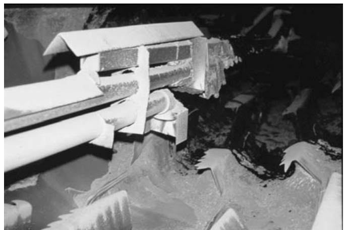
Figure 35. Typical location for introduction of fibers into drum-mix plant.
