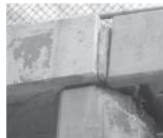
Bridge damage from magnitude 5.4 Chino Hills earthquake.
