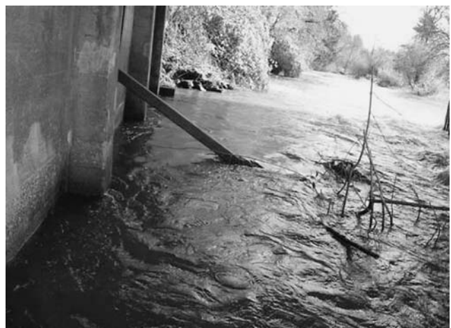
FIGURE 53 Debris build-up at sonar monitoring bracket on the Kline Bridge.
