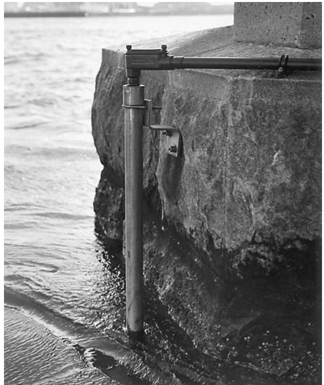
FIGURE 44 Detail of conduit to underwater sonar monitor, Robert Moses Causeway over Fire Island Inlet, Long Island.
