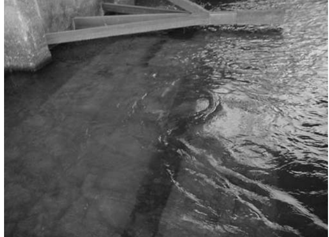
FIGURE 52 Scour monitor and concrete block rotation from continued scour near the Kline Bridge over Salmon Creek.
