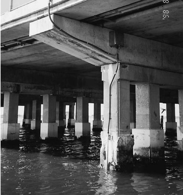
FIGURE 41 Remote station and conduit to sonar monitor at Wantagh Parkway over Sloop Channel, Long Island.
