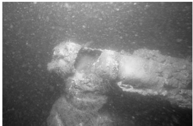
FIGURE F8 Damage due to corrosion and electrolysis.
