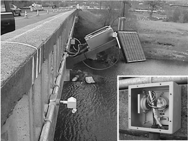
FIGURE 12 Tilt sensor installation with detail of the sensor.
