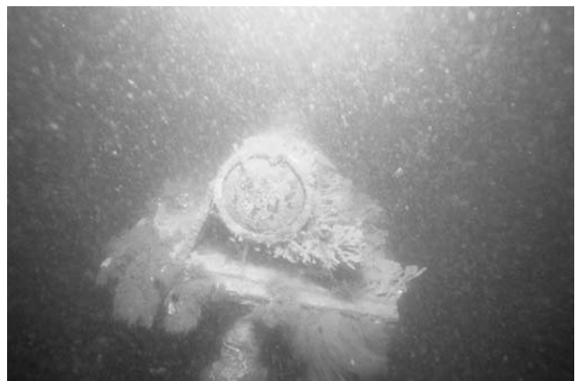
FIGURE 23 Underwater sonar bracket installation in the tidal environment showing the marine growth.
