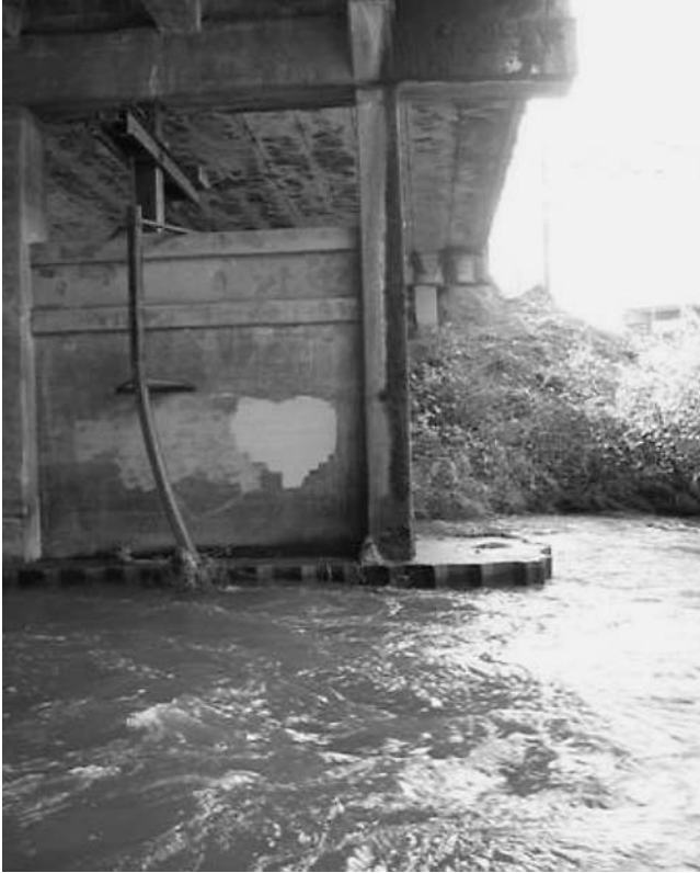
FIGURE 51 Conduit from sheet pile to tilt meter mounted on a pier of the Kline Bridge.
