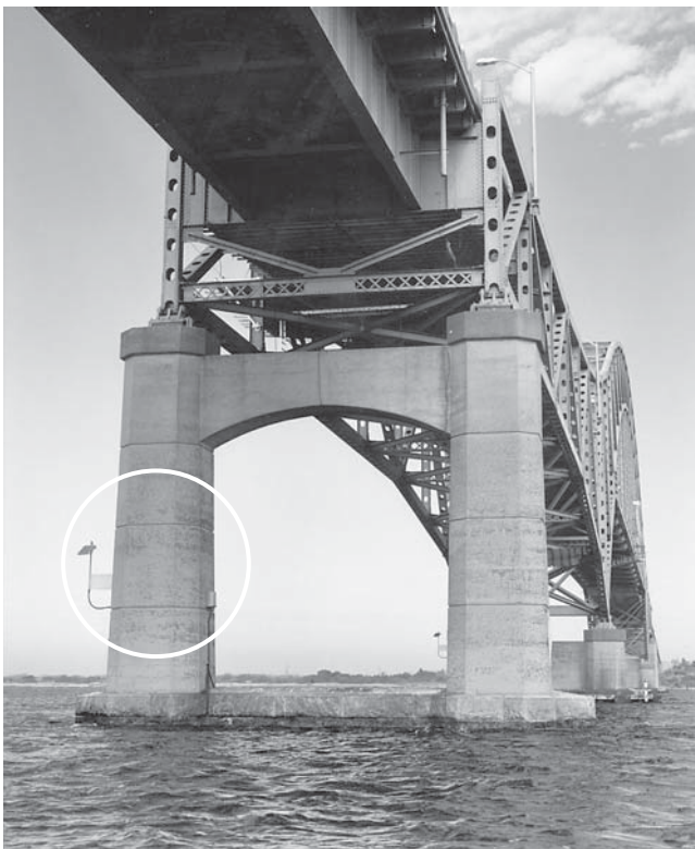
FIGURE 3 Scour monitoring system mounted on a pier on the Robert Moses Causeway over Fire Island Inlet, New York (circled) (Copyright: Raimondo di Egidio 2002).
