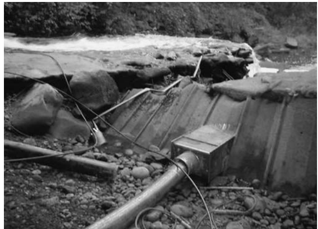
FIGURE 50 Tilt meter on downstream sheet pile to monitor the movement of the headcut toward the Kline Bridge over Salmon Creek.
