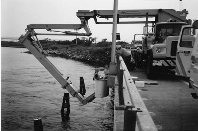
FIGURE 26 Installation of solar panels, remote stations, and conduit requires a snooper truck.
