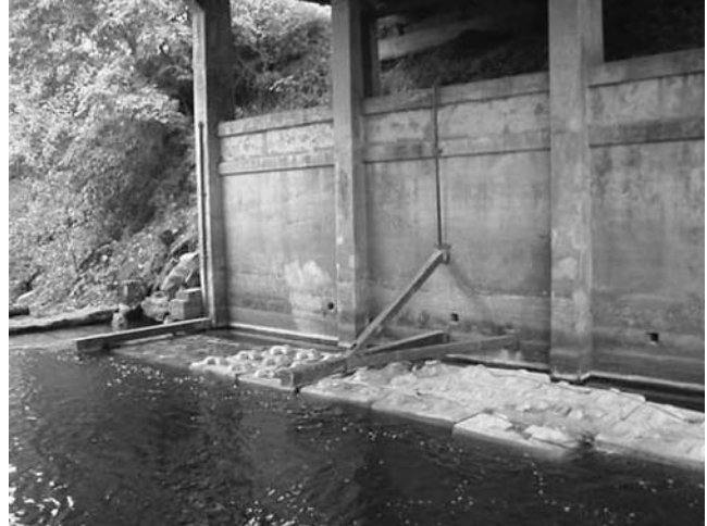
FIGURE 48 Two sonar scour devices monitor streambed elevations adjacent to the pier concrete block protection on the Kline Bridge.
