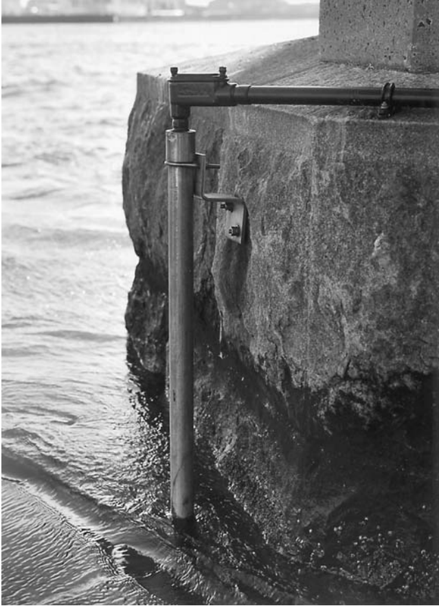
FIGURE 6 Detail of conduit to underwater sonar monitor (Copyright: Raimondo di Egidio 2002).
