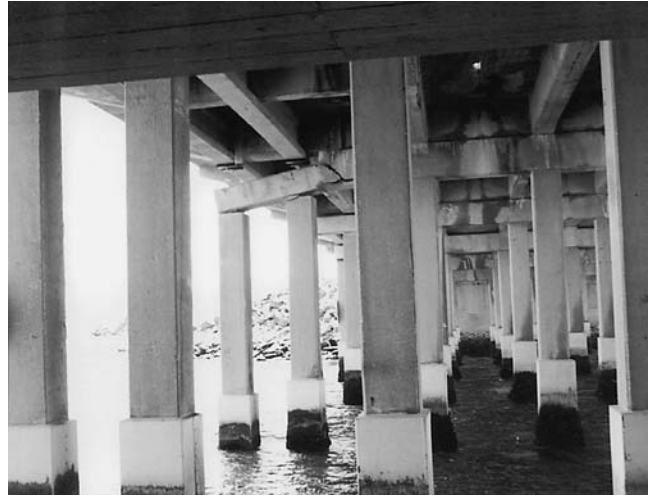
FIGURE F2 Failure of pier pile cap at Wantagh Parkway over Goose Creek.
