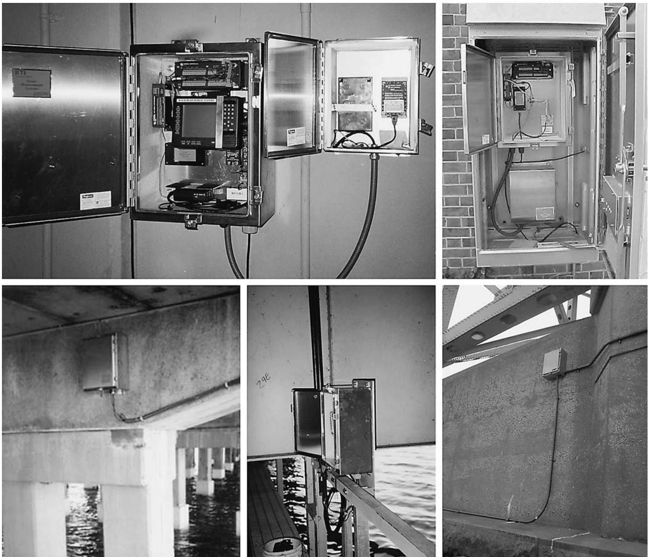
FIGURE 25 Locating the master and remote stations (clockwise from left to right). Master stations mounted inside a bascule pier machinery room and on a building near the bridge, remote stations on a pier stem, a catwalk under the bridge, and on a pier pile cap.
