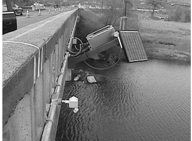
FIGURE 36 Tilt sensor installation on California bridge.
