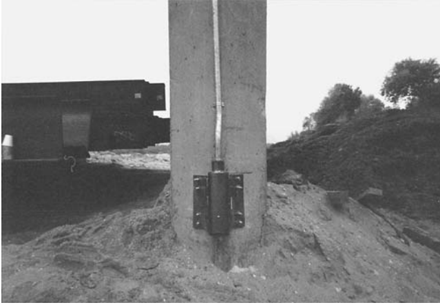
FIGURE 34 Close-up of sonar scour monitor installation on the Highway 101 Bridge over the Salinas River (Lagasse et al. 2001a).
