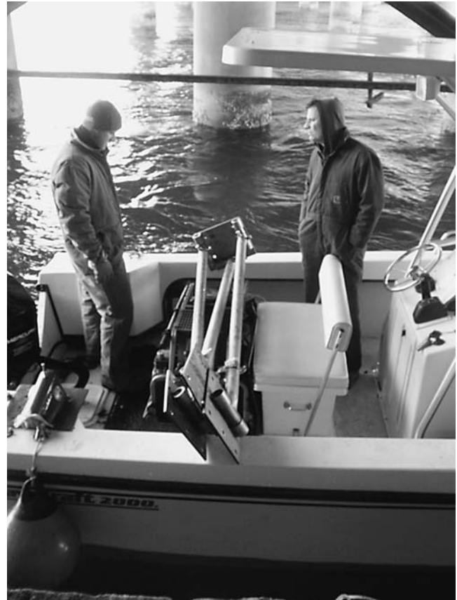
FIGURE 45 Adjustable sonar bracket prior to underwater installation on Wantagh Parkway over Goose Creek, Long Island.
