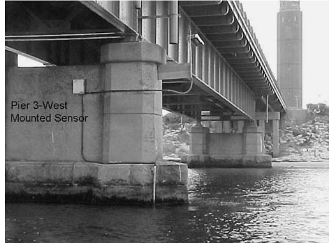
FIGURE 43 Remote station, solar panel, and conduit to sonar monitor for Robert Moses Causeway over Fire Island Inlet, Long Island (Copyright: Raimondo di Egidio).
