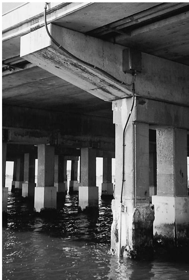
FIGURE F4 Scour monitoring system mounted to a pier on the Wantagh Parkway over Sloop Channel.
