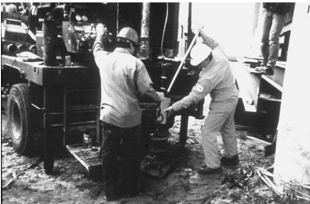
FIGURE 35 Installation of float-out devices with hand auger on the Highway 101 Bridge over the Salinas River (Lagasse et al. 2001a).
