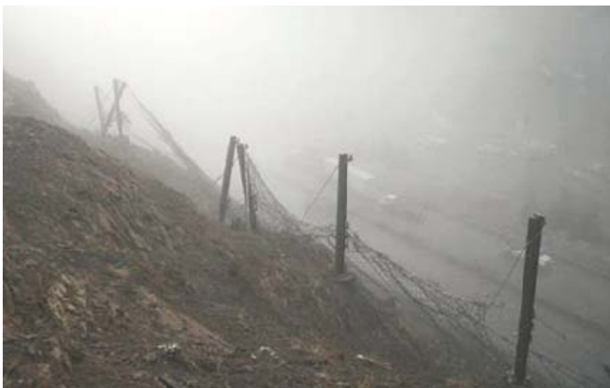
FIGURE 4 Damaged fence following April 2004 rockfall event.
