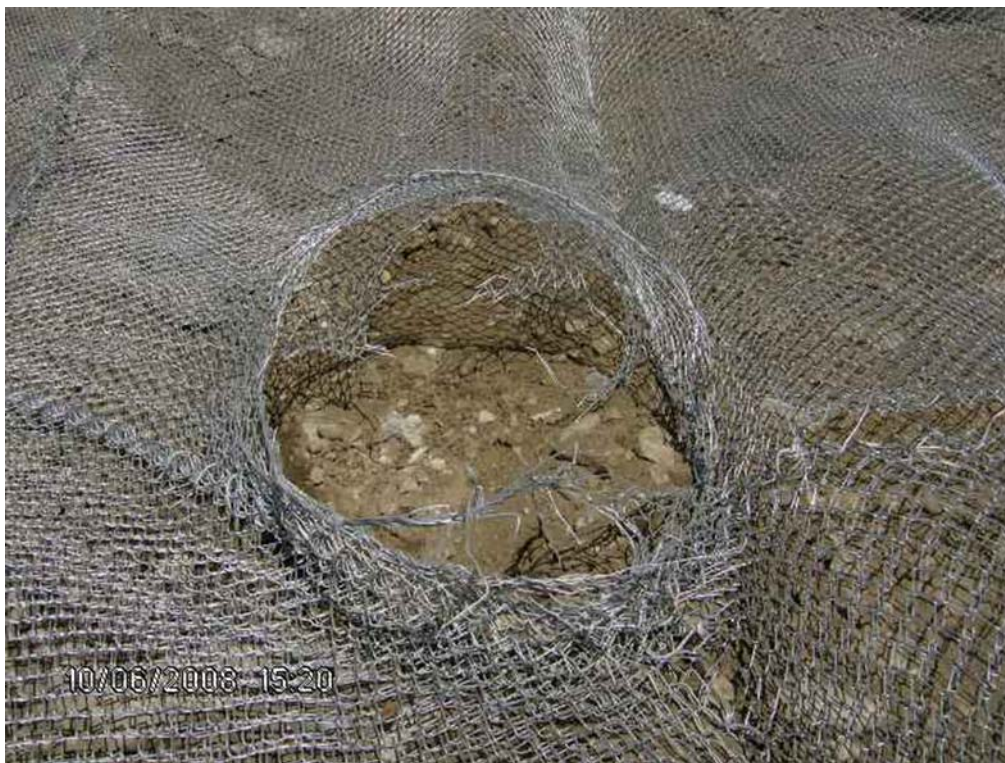
FIGURE 61 Severe damage to attenuator tail constructed with relatively light-weight, double-layer chain link mesh.
