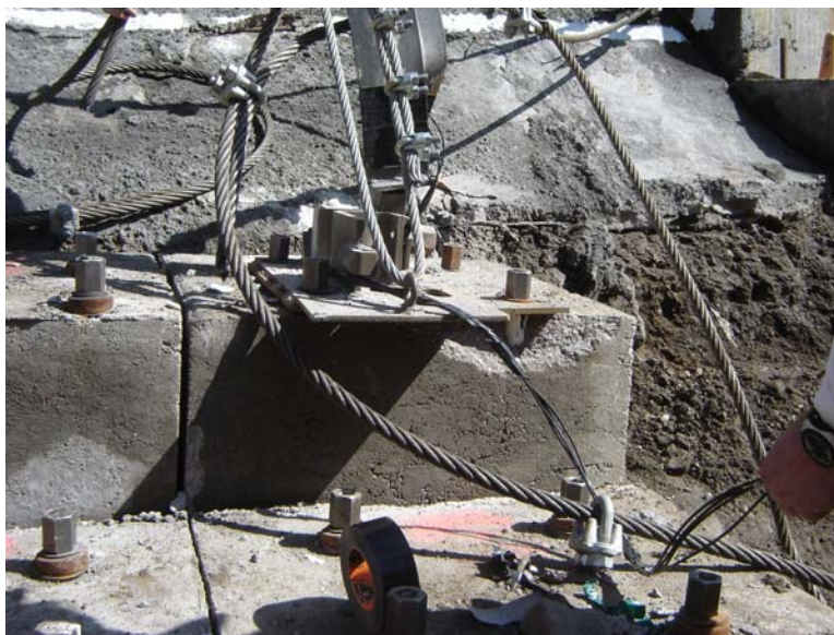
FIGURE 65 Minor concrete spalling as result of Test No. 120 (looking up ramp).
