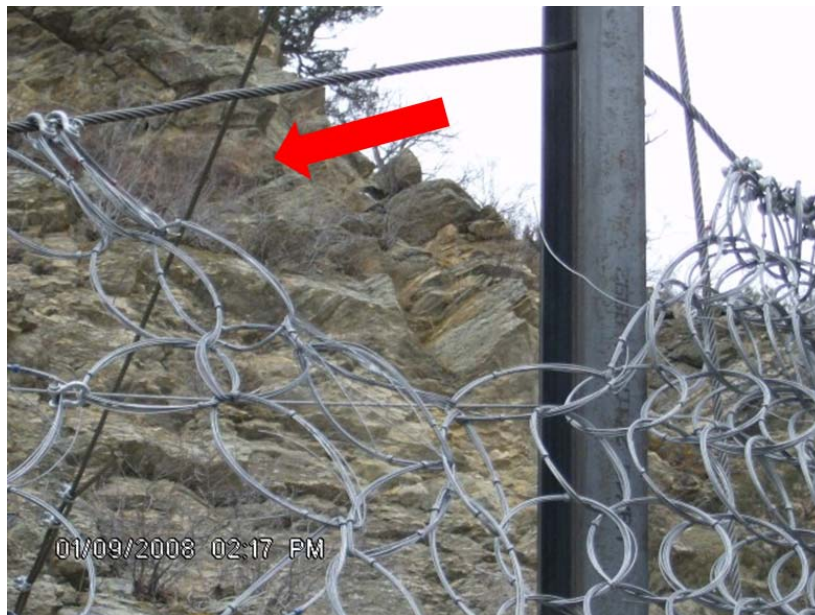
FIGURE 58 Bunching of ring net attached with shackles to support cable.
