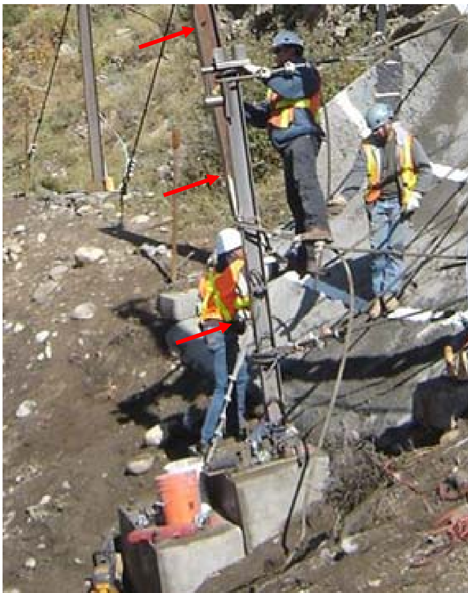
FIGURE 37 Pinned post attached to post foundation (arrows point to uphill anchor locations).
