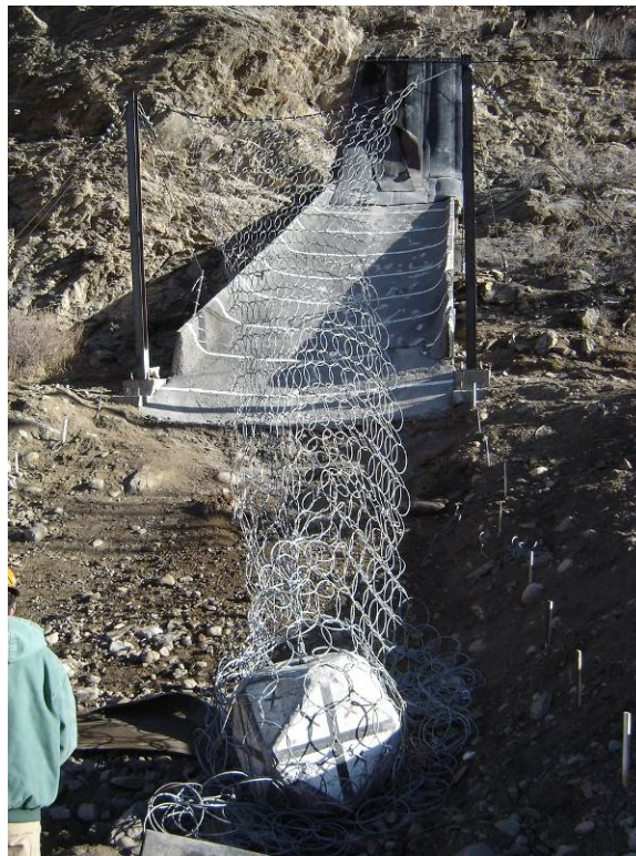
FIGURE 42 Example of single-panel system wrapping and entangling a rock.
