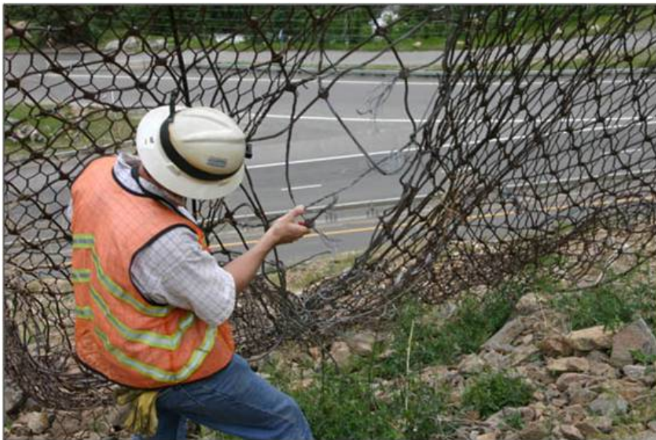
FIGURE 8 Damage to prototype attenuator at Georgetown (damage caused by either stretching or cutting of 8-mm wire rope cable net).
