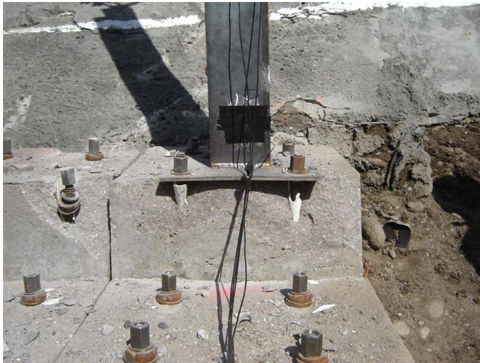
FIGURE 69 Fixed connection post base placed on same base for Test No. 120 (concrete spalling after Test No. 122 looking up ramp).
