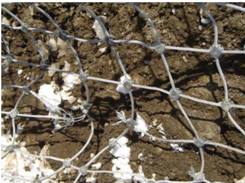
FIGURE 56 Significant damage to 8-mm cable net constructed with interlocking clips.
