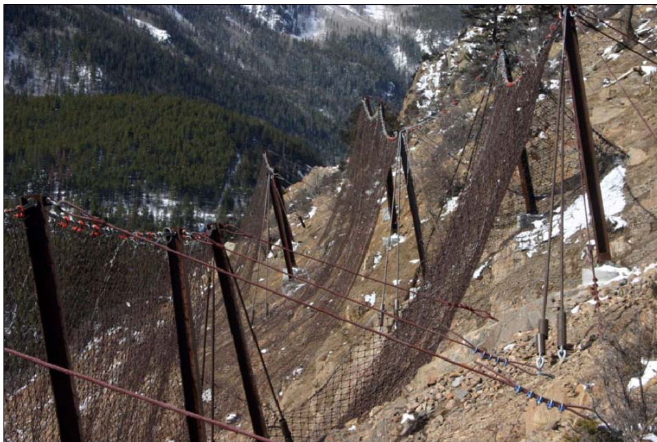
FIGURE 6 View of prototype attenuator system installed above Georgetown Incline.
