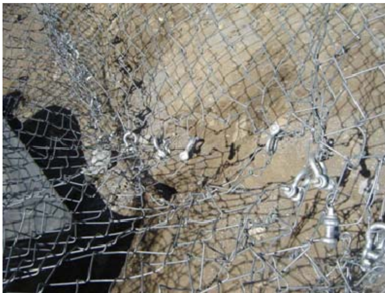
FIGURE 55 Stretching and damage along seam of 4-mm high-tensile-strength wire net.
