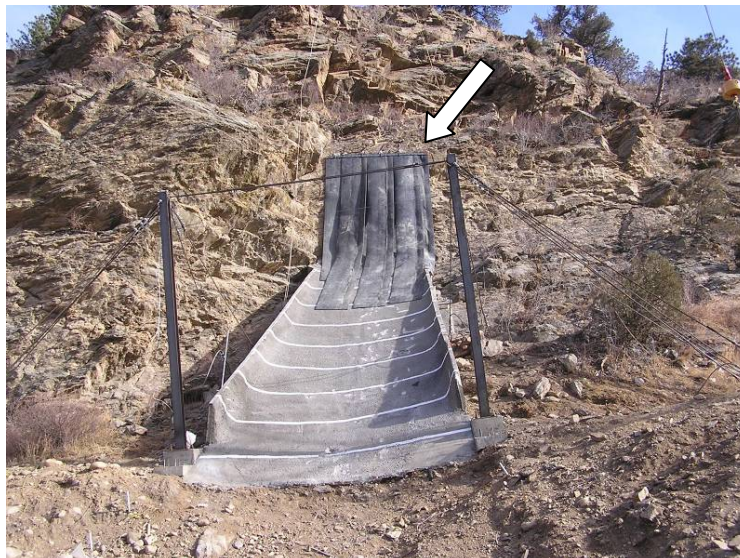
FIGURE 14 Rubber conveyor belts (trimmed to top of concrete ramp prior to testing) were used to protect rock face from impact damage (arrow depicts top of conveyor).
