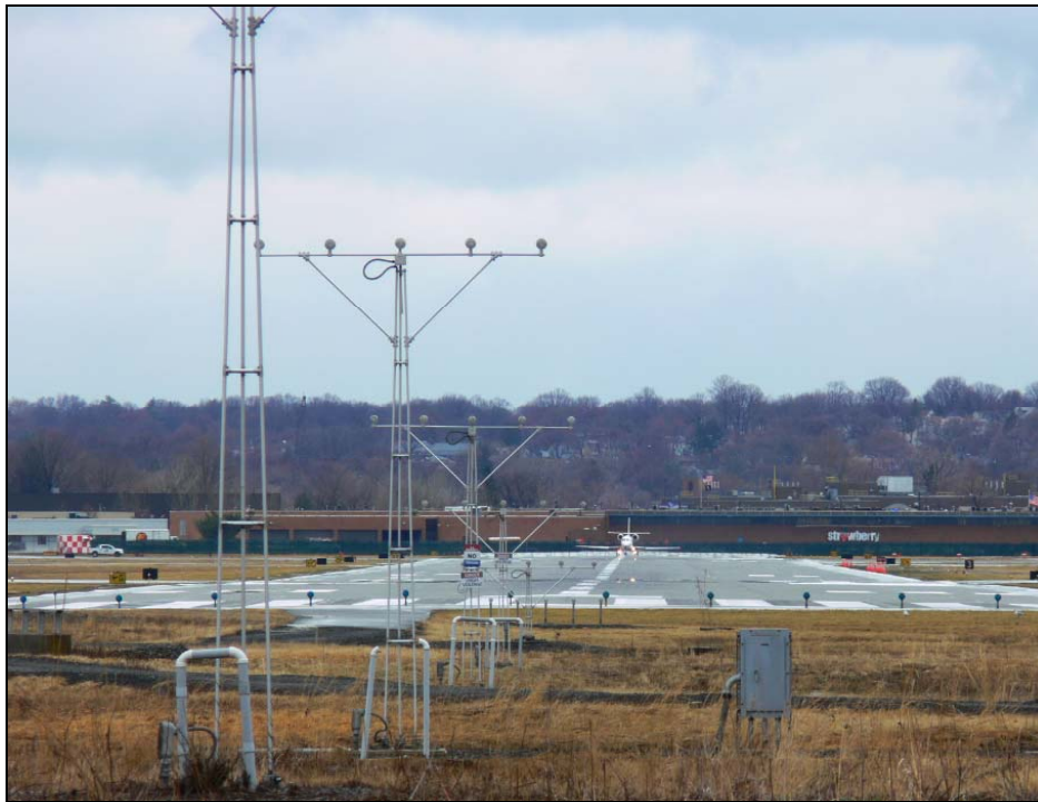
Figure 10. Approach Lights Mounted on Aluminum Lattice Support Structures
