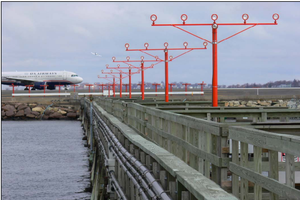
Figure 12. Approach Lights Mounted on Hybrid Supports (Frangible Fiberglass Tubular Poles and Non-frangible Wooden Pier Structure): Over-the-water Pier Installation
