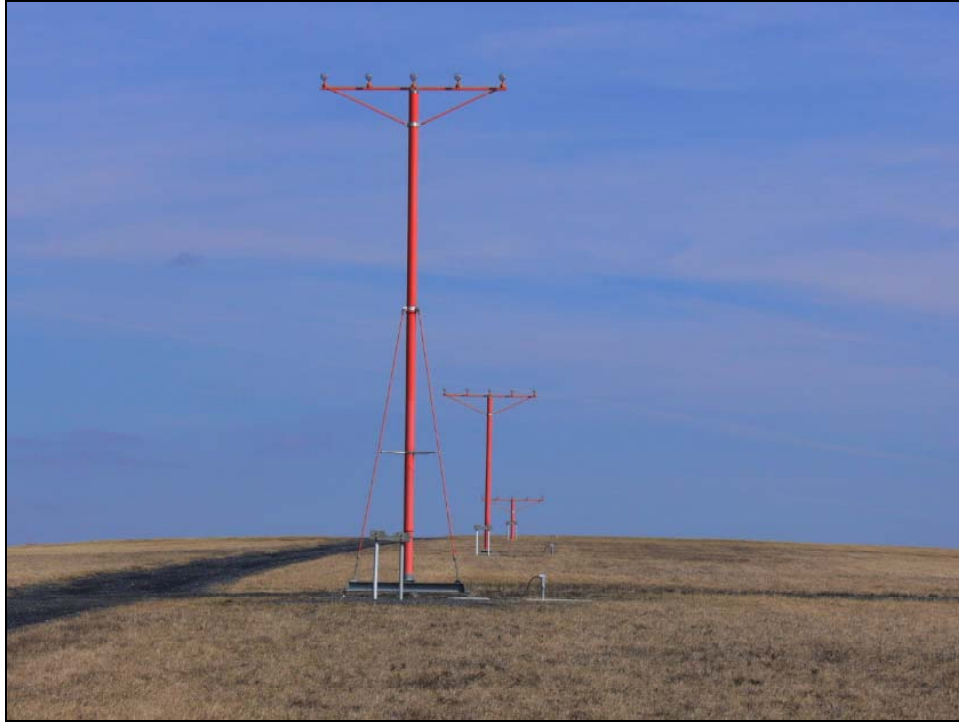
Figure 9. Approach Lights Mounted on Fiberglass Tubular Poles
