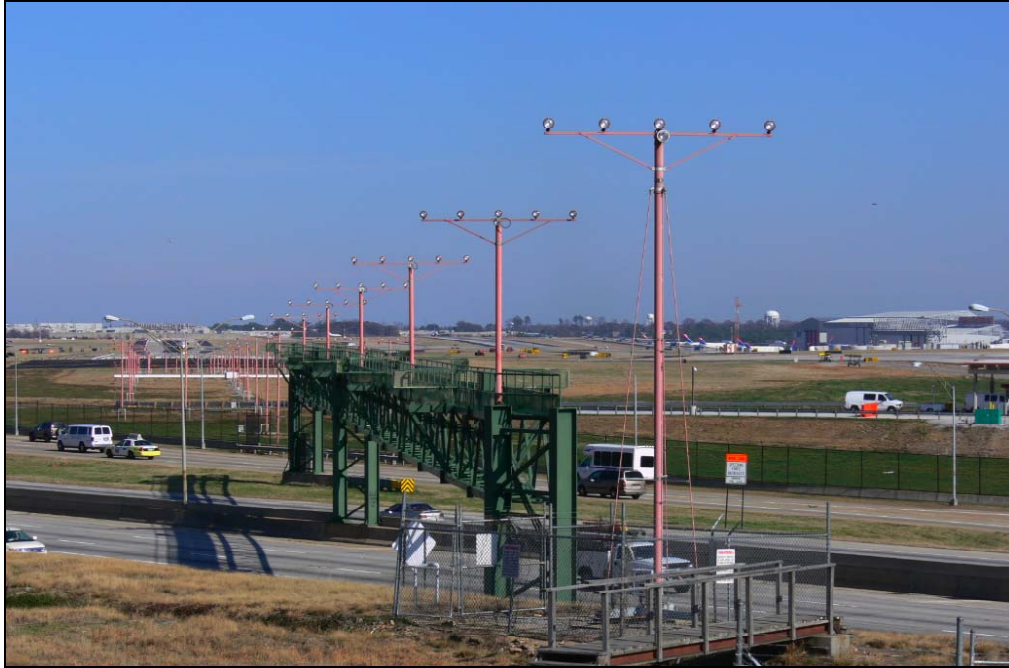
Figure 11. Approach Lights Mounted on Hybrid Supports (Frangible and Non-frangible): Land Installation
