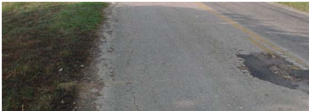
FIGURE 3 Narrow pavement creates edge problems.
