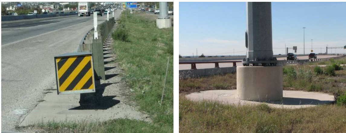
FIGURE 13 Good mow strips under rail and around luminary.
