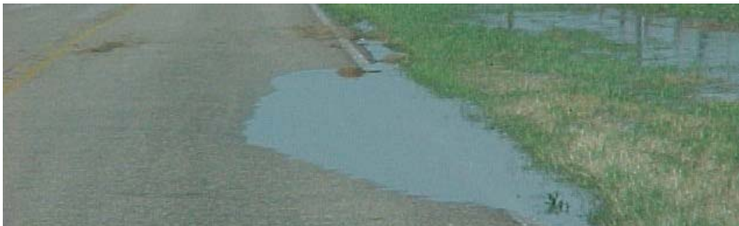
FIGURE 1 Inadequate ditch forces water onto the pavement.
