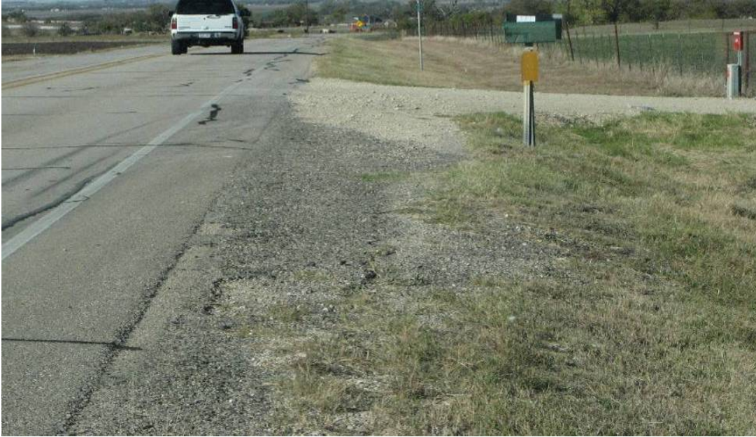
FIGURE 14 Mailbox turnout with rap installed to eliminate water standing area.
