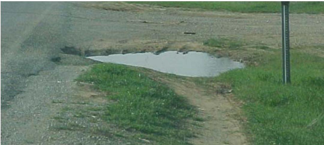
FIGURE 15 Water standing where no turnout is installed.
