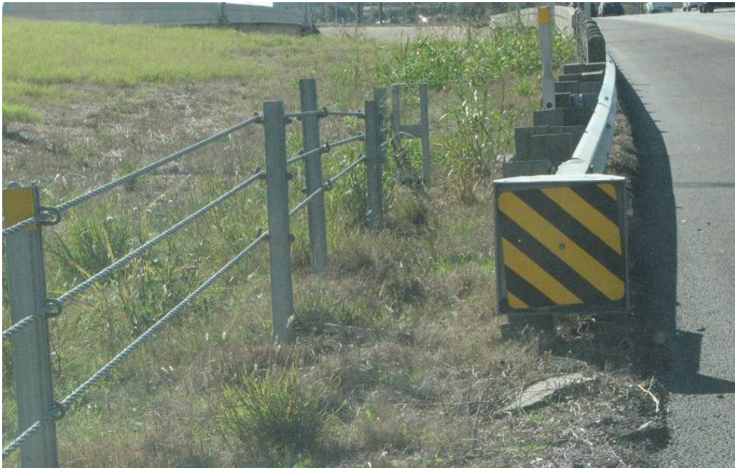
FIGURE 11 Cable barrier terminates behind guardrail, creating inaccessible area.
