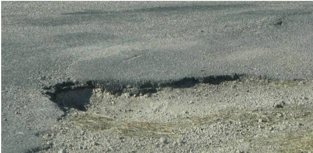
FIGURE 16 Unmaintained driveway provides location for water to get into roadway base.
