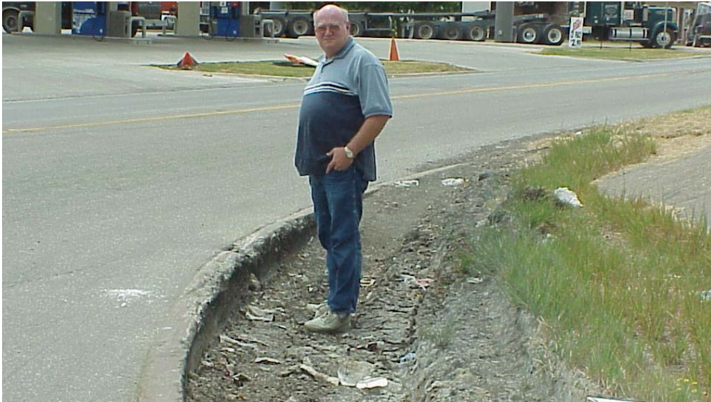
FIGURE 2 Truck traffic has created a severe rut along pavement, even behind curb.
