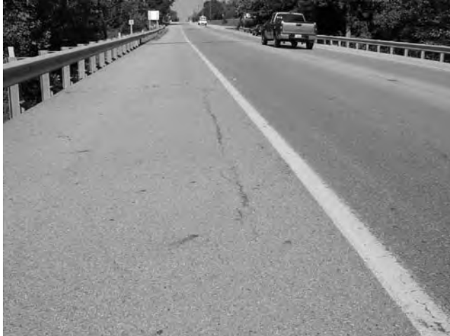
FIGURE 18 Longitudinal cracking in asphalt riding surface (Source: Henry G. Russell).
