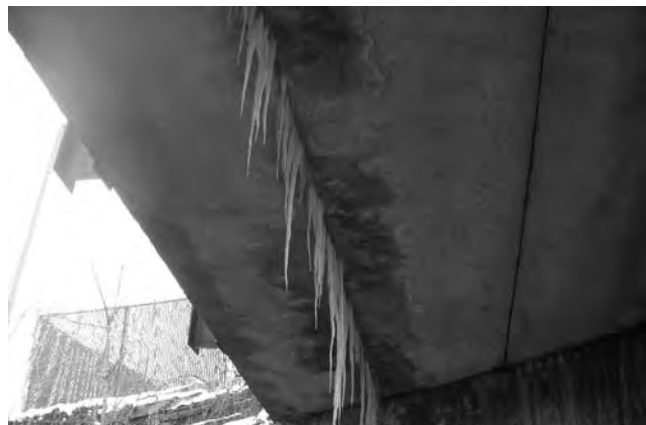
FIGURE 20 Leakage through longitudinal joints (Source: Pennsylvania DOT).
