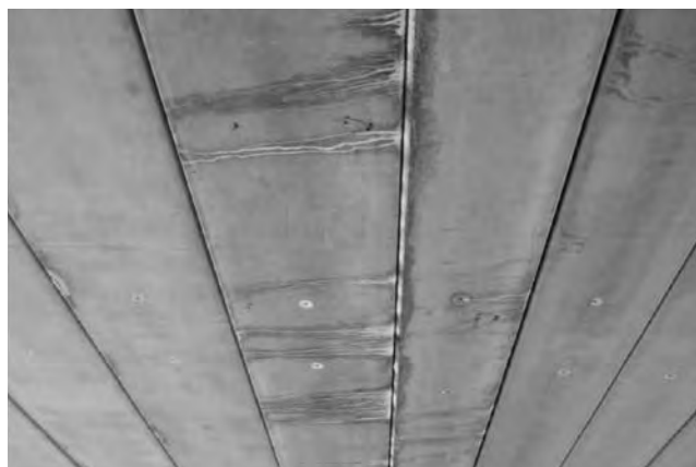
FIGURE 21 Efflorescence on the underside, indicating leakage through the joints (Source: New York State DOT).
