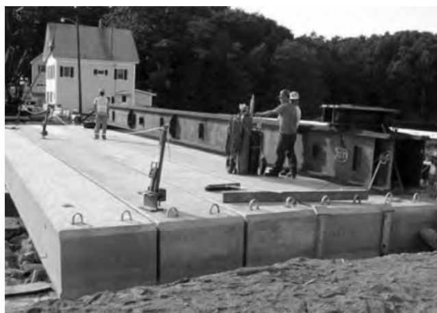
FIGURE 4 Adjacent box beams used for the superstructure of the Davis Narrows Bridge, Maine (Source: Maine DOT).
