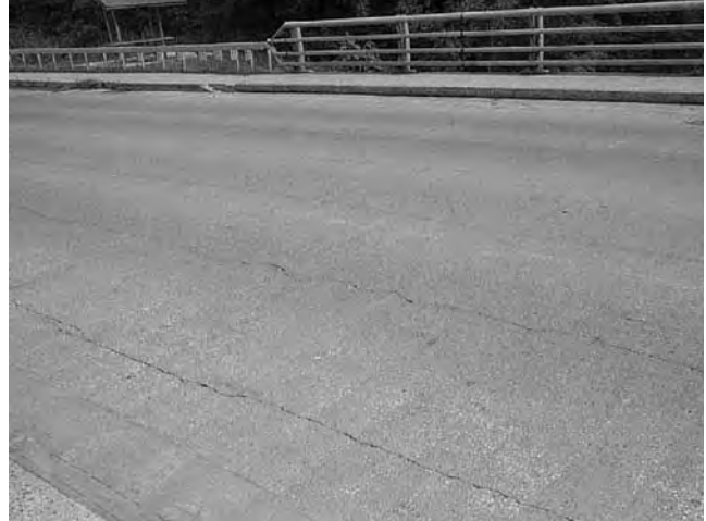
FIGURE 19 Longitudinal cracking in composite concrete deck (Source: New York State DOT).
