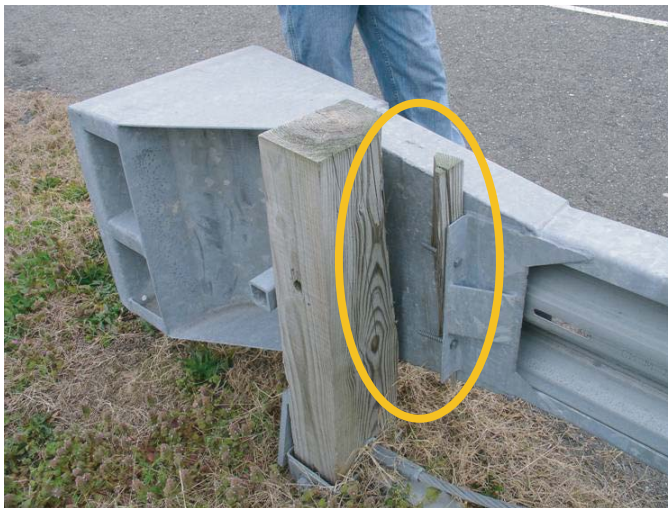
Figure 68. Failed attachment of lag bolts to end post.
