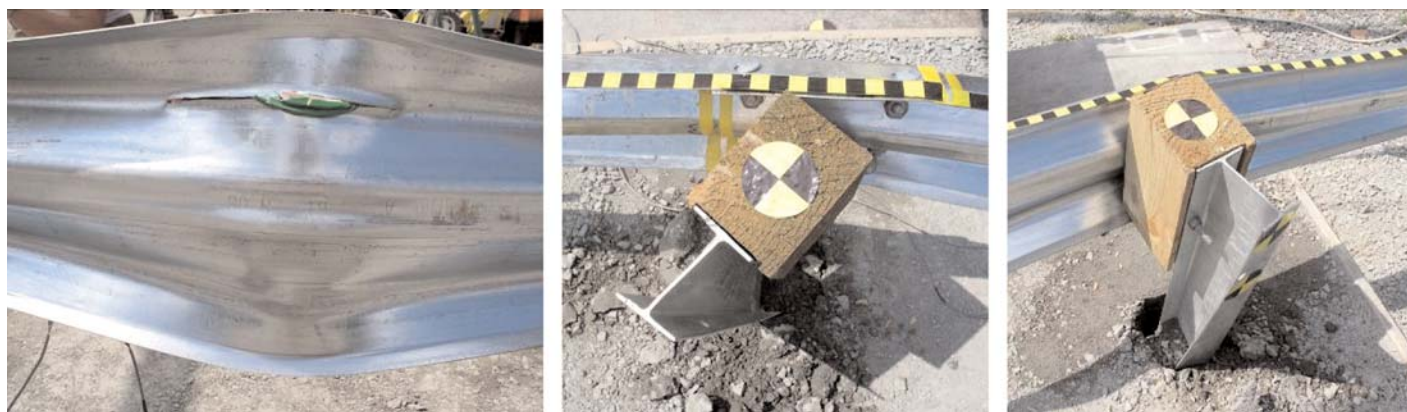
Figure 20. Test 07-3: detailed view of impact location (left), post damage at splice (center), and non-splice location (right).
