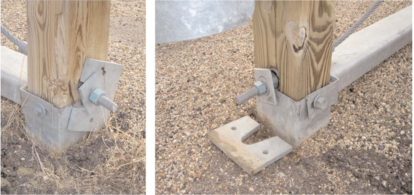
Figure 65. Misaligned or missing bearing plates (photo: courtesy of South Dakota DOT).
