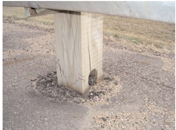
Figure 64. Wood post with cross-grain cracking (photo: courtesy of South Dakota DOT).
