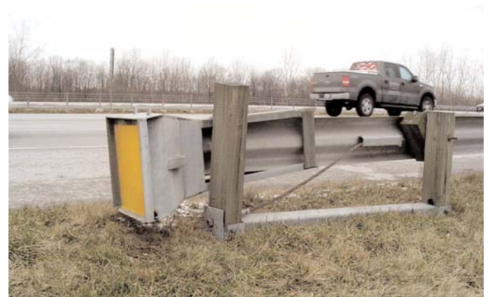
Figure 67. Misaligned impact head because of missing lag bolts (photo: courtesy of Ohio DOT).
