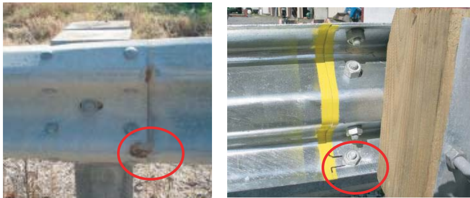
Figure 23. Splice damage evaluated in pendulum tests.
