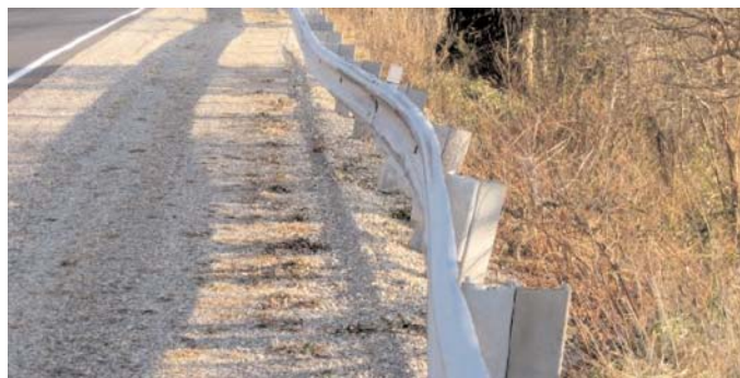
Figure 37. Guardrail with rail and post deflection.
