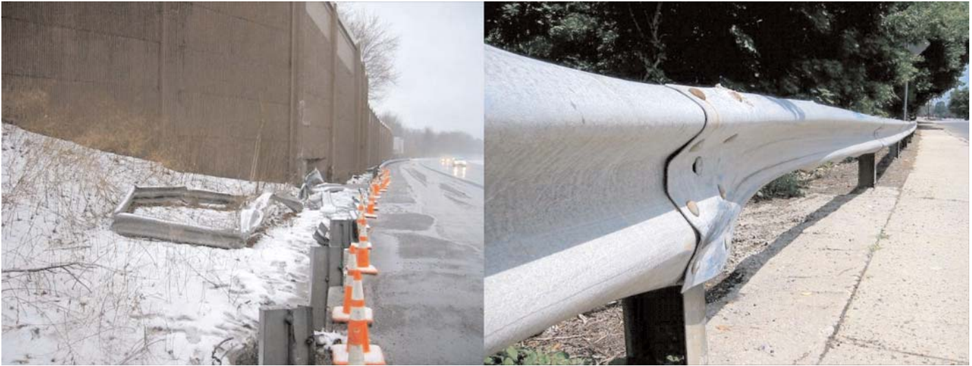
Figure 1. Catastrophic vs. minor guardrail damage.
