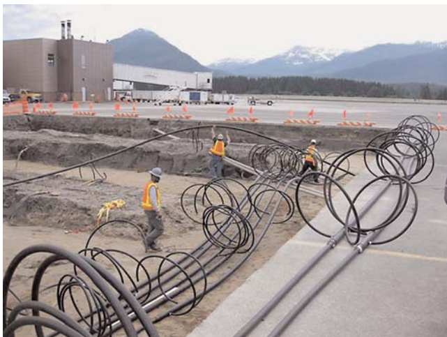
FIGURE 12 Geothermal well field. Well fields installed below existing pavements at Juneau International Airport (Courtesy: JNU).
