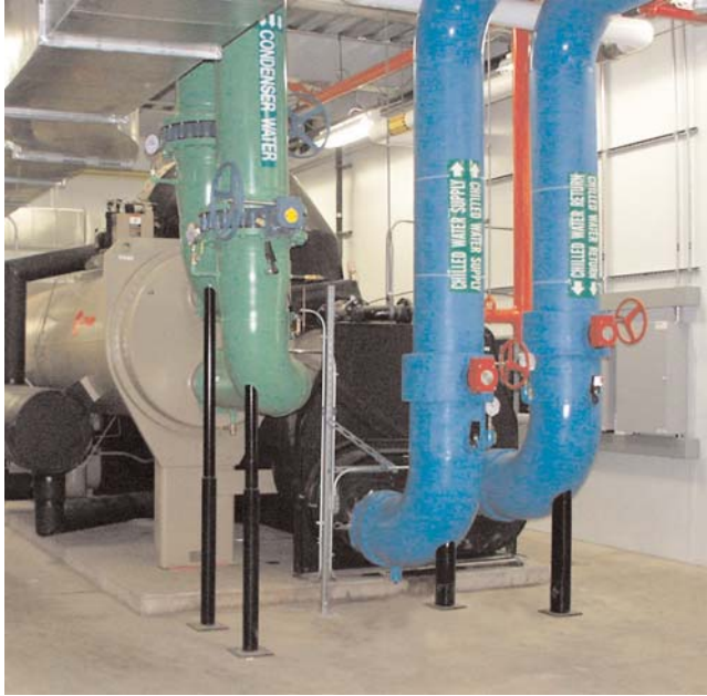
FIGURE 9 Central chiller replacement. Chiller and condenser upgrades at MSP Lindbergh Terminal. (Courtesy: Michaud Cooley Erickson Engineers.)
