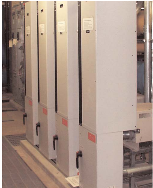
FIGURE 3 Motor controls. Variable frequency drives for condenser water pumps save energy at MSP Airport. (Courtesy: Michaud Cooley, Erickson Engineers.)
