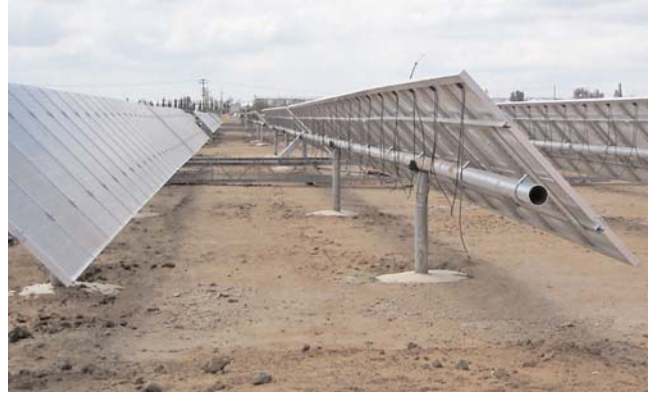
FIGURE 8 Photovoltaic panels and supports at Fresno Yosemite International. (Courtesy: Fresno–Yosemite International Airport.)
