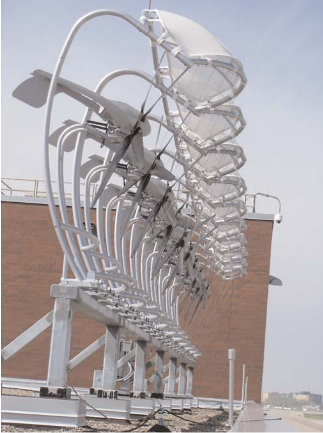
FIGURE 14 Micro scale wind turbines. Parapet mounted turbines mounted on the airport fire station at MSP.
