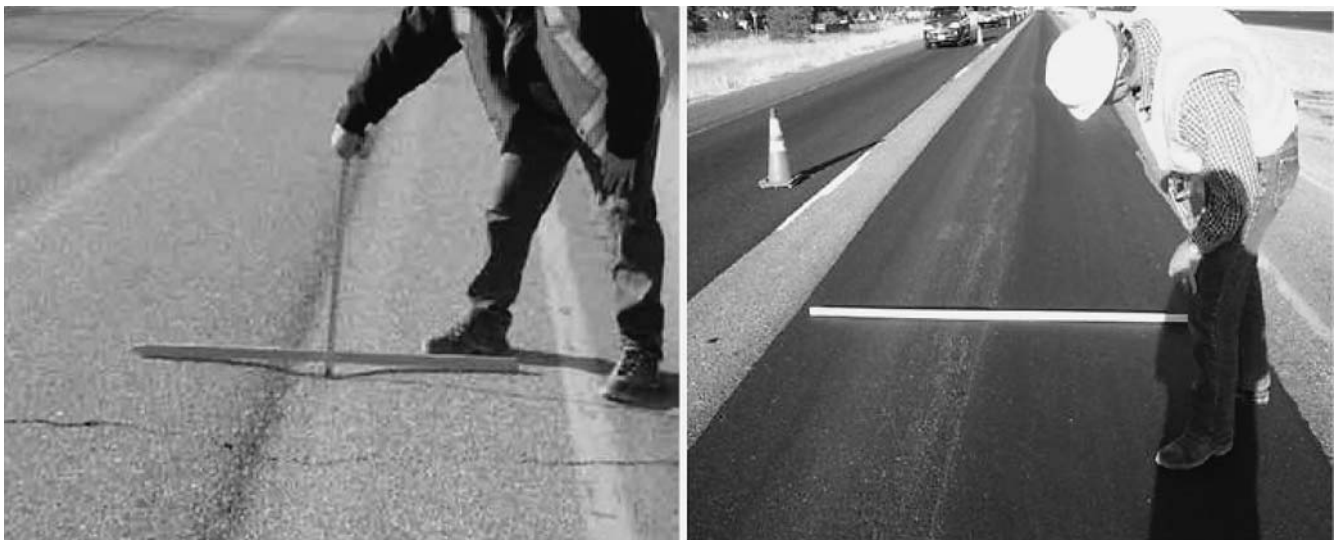
FIGURE 21 Microsurfacing applied to rutting caused by studded tires in Washington State: before and after (Washington State DOT 2009).
