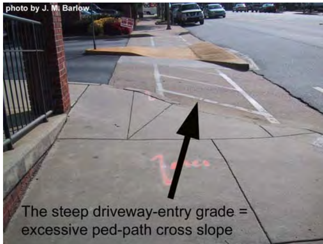
EXHIBIT 3-9 Excessive sidewalk cross slope at driveway
