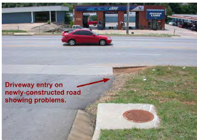
EXHIBIT 3-5 Indicators of problems with driveway entry geometry
