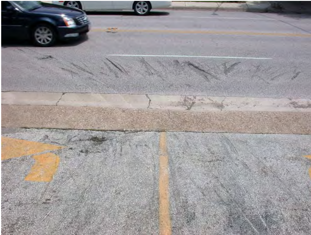
EXHIBIT 4-5 Example of a driveway with visible vehicle underside scrape marks
