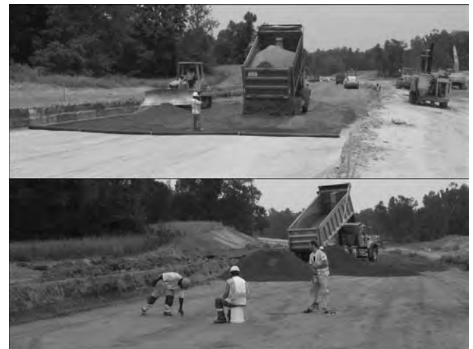
Figure 8.28. Placing material (top) and performing spot-test measurements (bottom) in an active Evaluation Section at the North Carolina work site.
