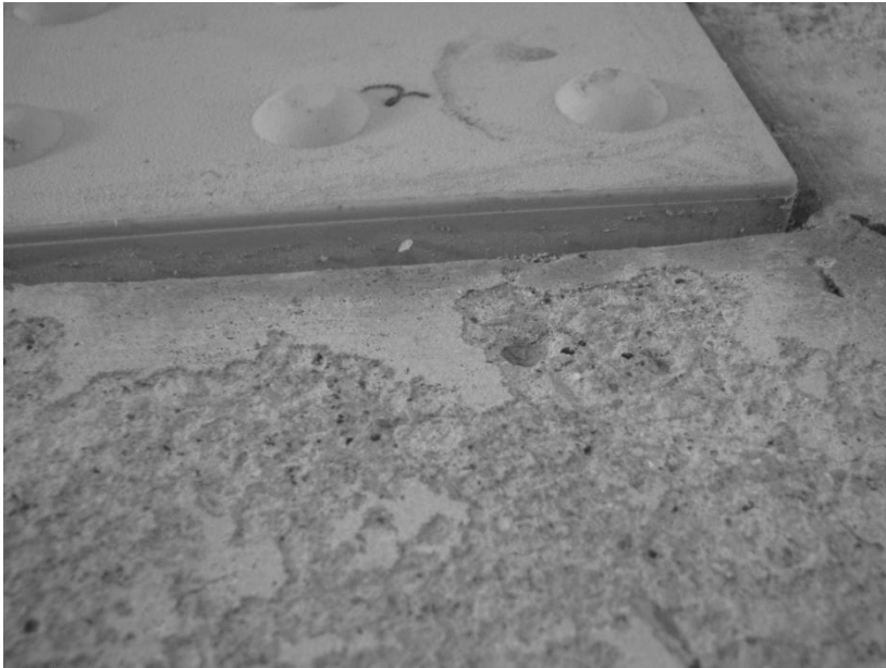
Figure 5 - Relative displacement of a detectable warning system, caused by freeze jacking.
