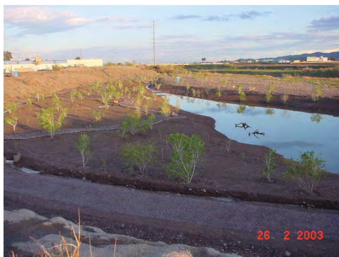
This Army Corps of Engineers river channel restoration project is less than 650 ft from runway centerline at a major airport. Airport managers must work with the Corps to protect airport airspace and aviation safety. (Photo courtesy USDA)
