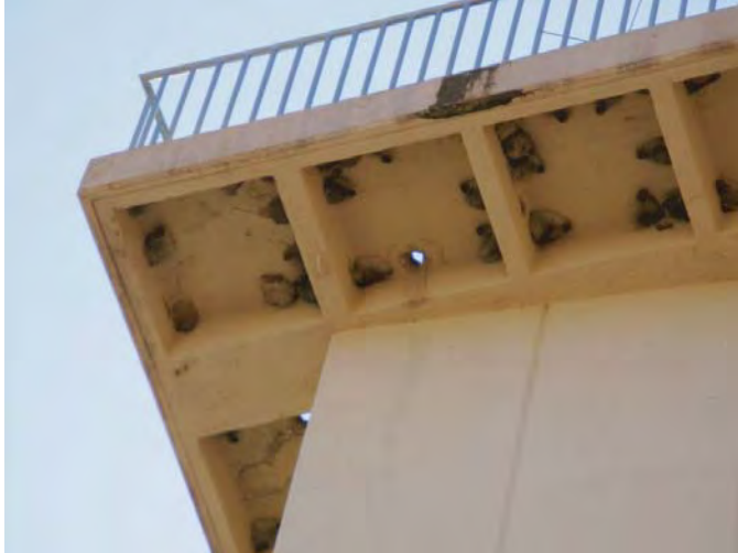
These swallow nests are under the air traffic control tower's upper exterior catwalk. Active nests are protected and a federal depredation permit is needed before they may be taken. (Photo E. Garcia)
