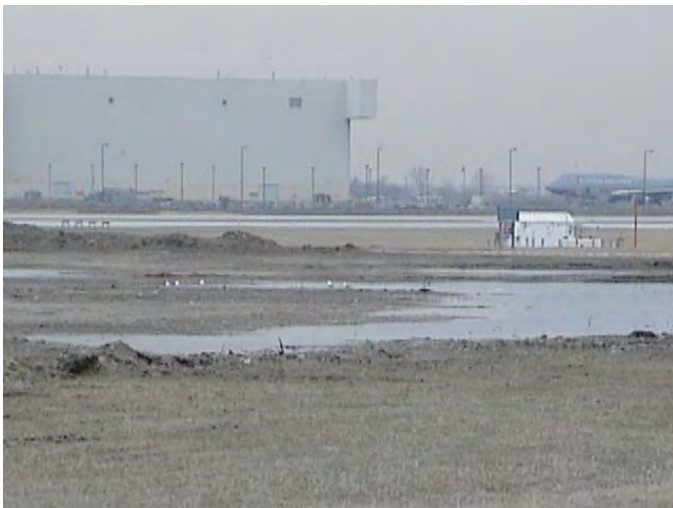
Standing water can be very attractive to birds. This is a construction site at a midwestern airport. (Photo courtesy FAA)
