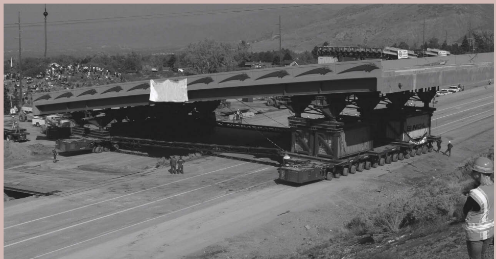
Crews used an SPMT to move the 4500 South Bridge superstructure from the construction site to its final location over Interstate 215.
