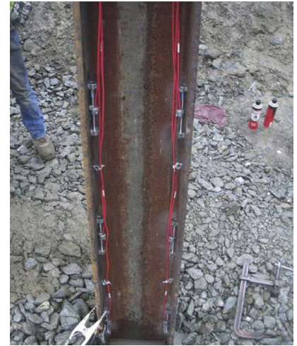
Strain gauges ( left ) close up and ( right ) installed on H-piles for Middlesex Bridge.
