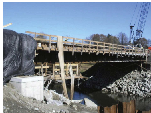
The 37-meter-long East Montpelier Bridge is part of ongoing research to establish design guidelines for integral abutment bridges.
