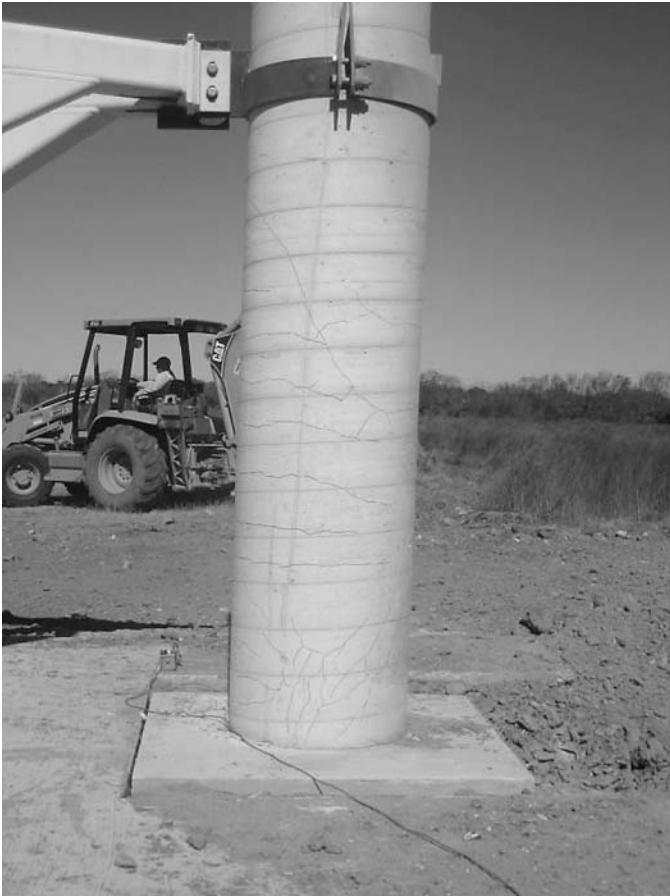
Figure 57. Small standoff blast damage: Column 2-Seismic.
