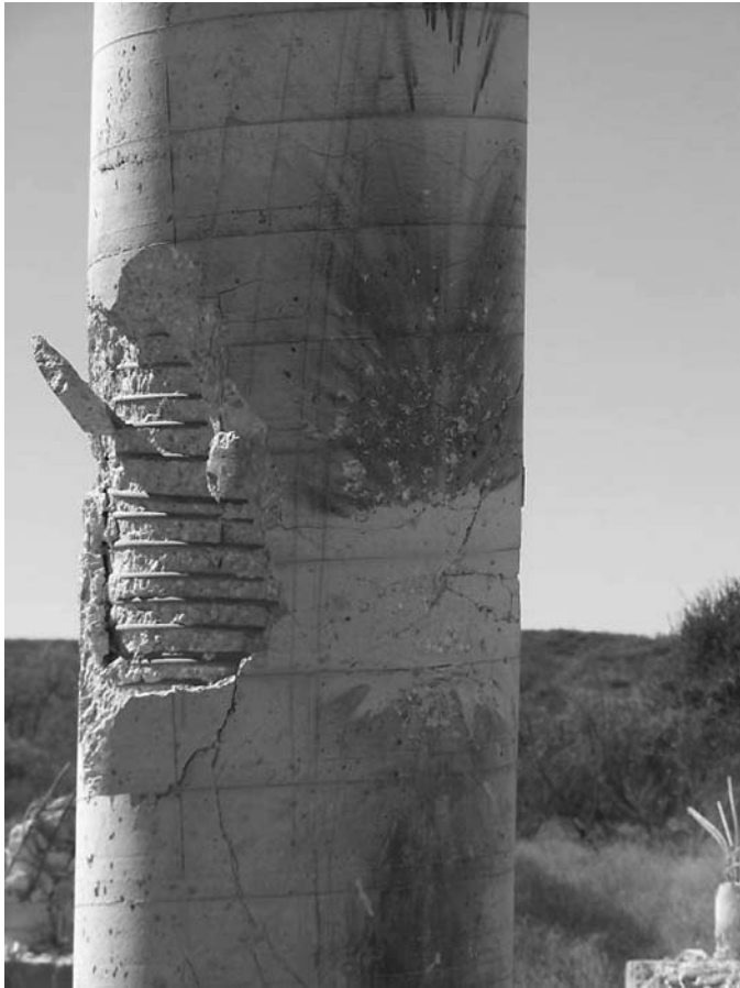
Figure 65. Local damage Test 5: Column 2-Blast.
