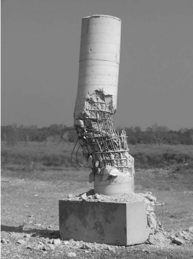
Figure 62. Local damage Test 2: Column 2A1.
