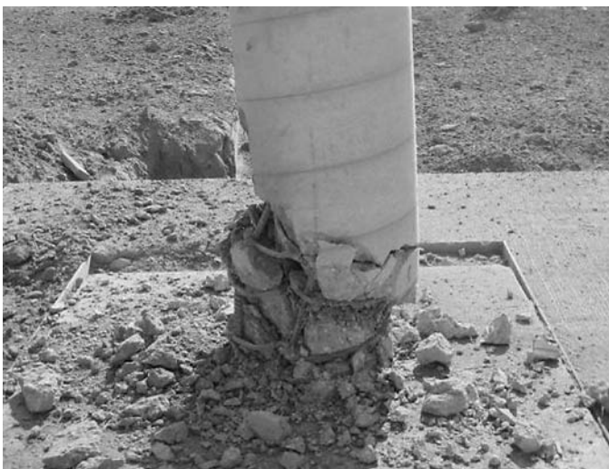
Figure 78. Direct shear failure.
