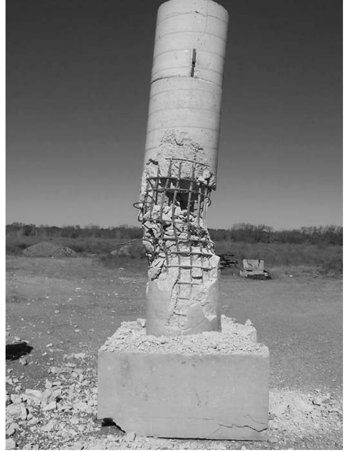
Figure 64. Local damage Test 4: Column 2B.
