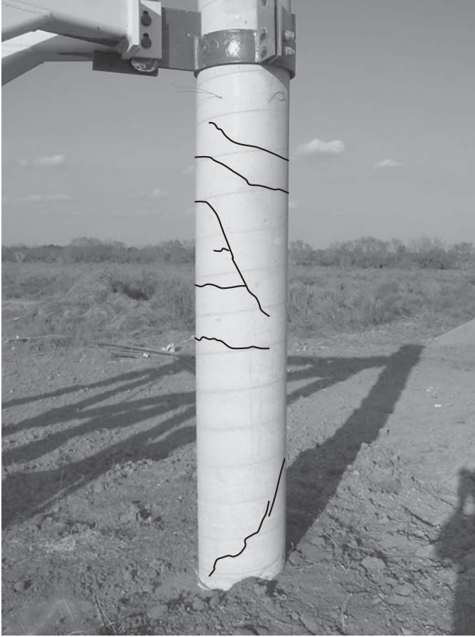
Figure 51. Small standoff blast damage: Column 1A1.
