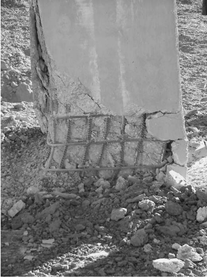
Figure 59. Small standoff blast damage: Column 3A.
