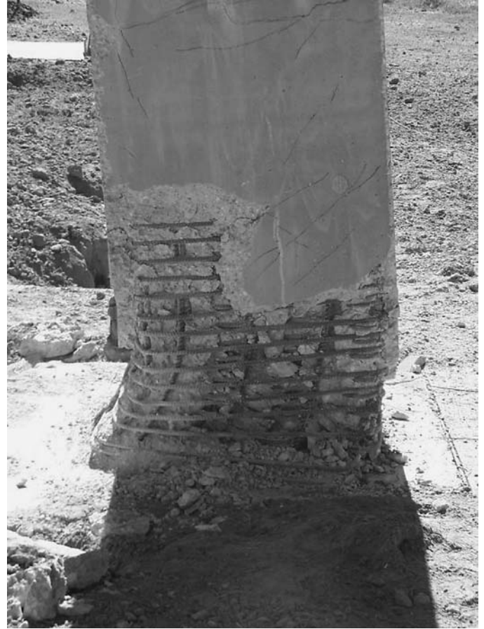
Figure 60. Small standoff blast damage: Column 3-Blast.
