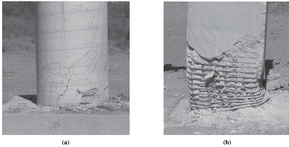
Figure 74. Columns meeting minimum transverse reinforcement requirements: a) minor damage (2-Blast), b) extensive damage (3-Blast).
