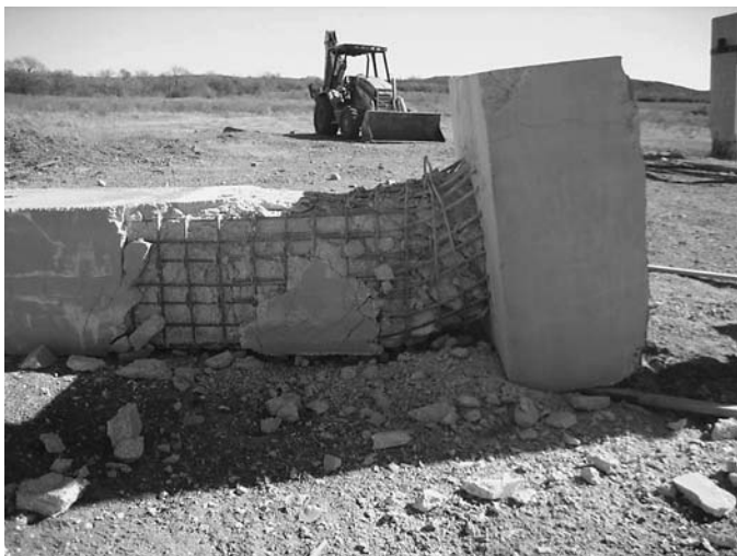
Figure 66. Local damage Test 6: Column 3A.
