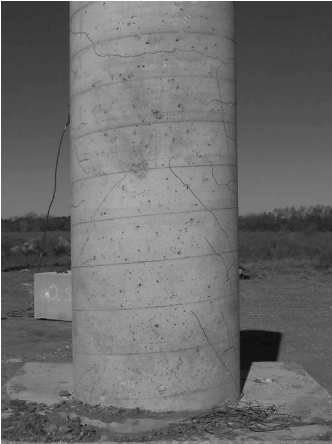
Figure 56. Small standoff blast damage: Column 2B.
