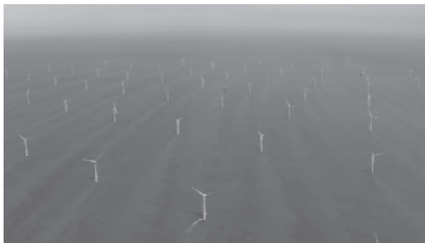
FIGURE 2-7 300-MW Thanet wind project off the southeast coast of England. (SOURCE: Vattenfall; photograph by Lavernder Blue.)
