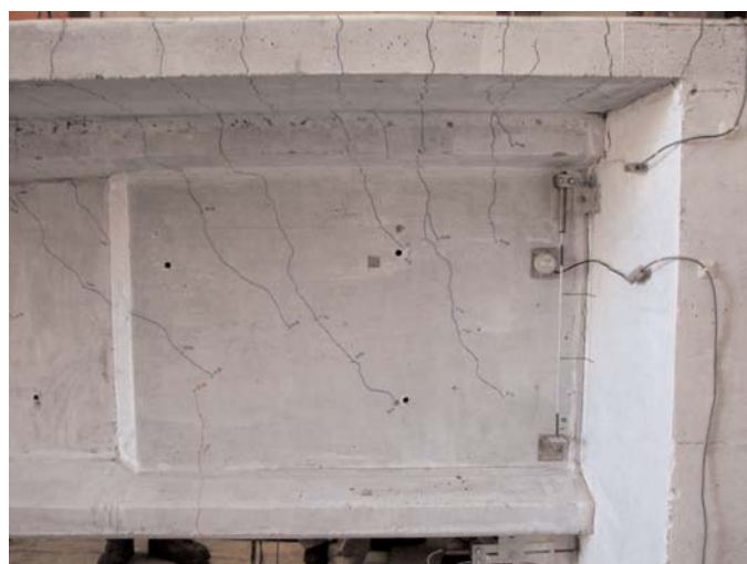
Figure 2.83. Girder end block region at -0.29\% joint rotation.
