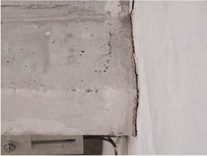
Figure 2.84. Girder bottom flange joint opening at +0.19% joint rotation.
