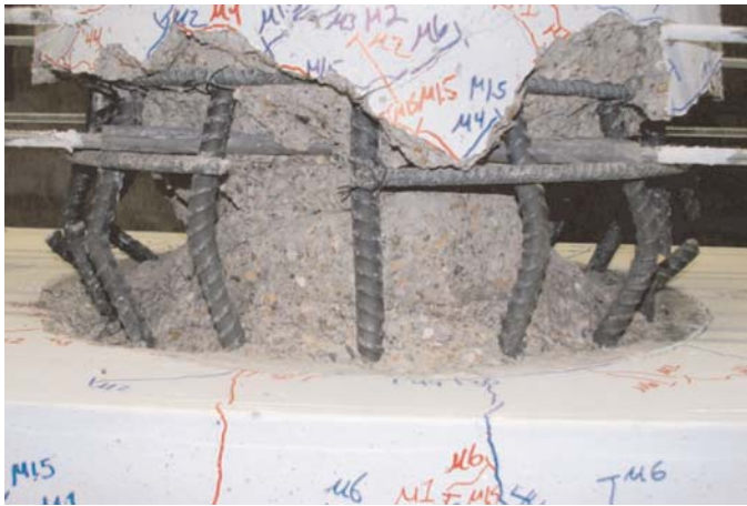
Figure 3.7. View of column bar buckling at interface between the bent cap and column—CPFD (after removal of concrete post-test).
