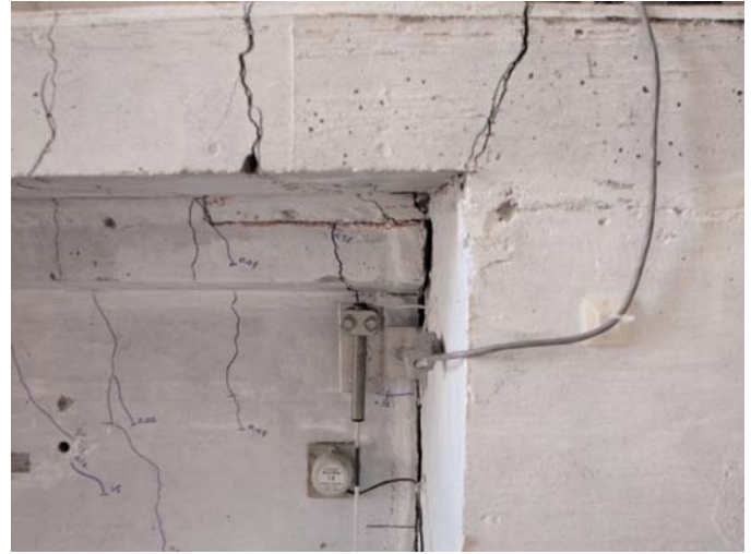
Figure 2.85. Girder to deck interface crack at -0.79% joint rotation.
