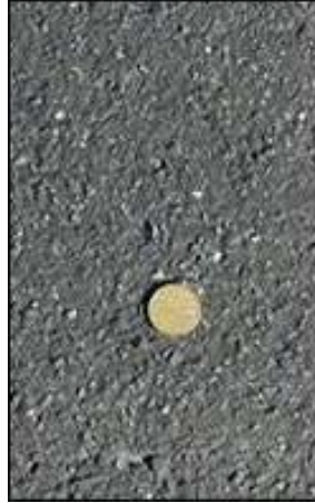
FIGURE B2 Microsurfacing texture one year after construction; diameter of the coin is 1 in.
