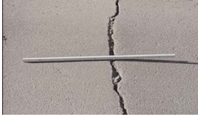
FIGURE B4 Transverse crack heaving caused by water that saturated pavement structure and froze.
