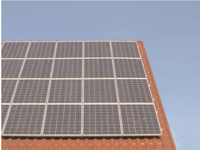
FIGURE 1 Solar PV on roof [courtesy: Harris Miller Miller & Hanson Inc. (courtesy: HMMH)].
