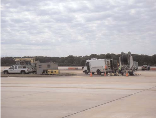
FIGURE 29 Airfield construction project. Source: F. Dettmann, A.A.E., Hillsborough County Aviation Authority, Tampa International Airport.
