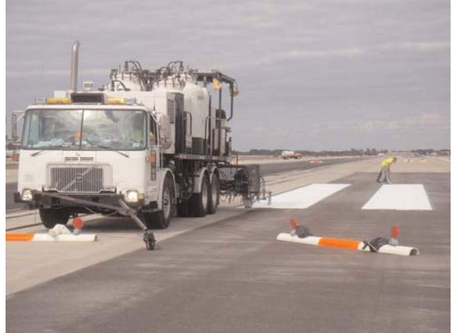
FIGURE 19 Newly painted markings. Source: F. Dettmann, A.A.E., Hillsborough County Aviation Authority, Tampa International Airport.
