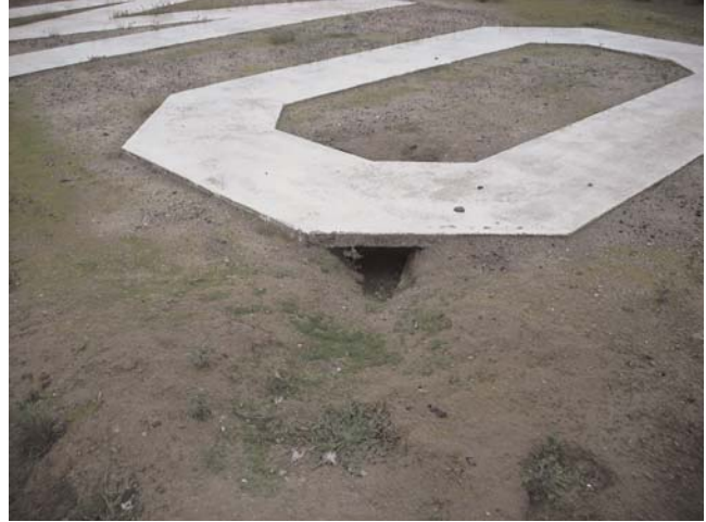
FIGURE 15 Safety area rut and exposed concrete base. Source: Lammerding 2010a.
