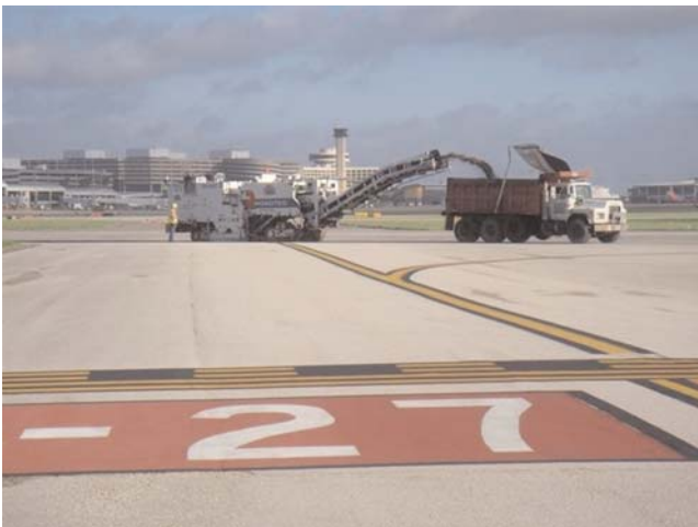
FIGURE 30 Airfield construction project. Source: F. Dettmann, A.A.E., Hillsborough County Aviation Authority, Tampa International Airport.
