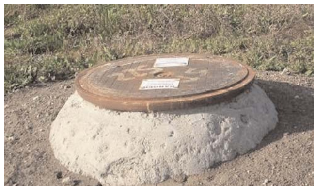
FIGURE 16 Safety area manhole above grade. Source: Lammerding 2010b.
