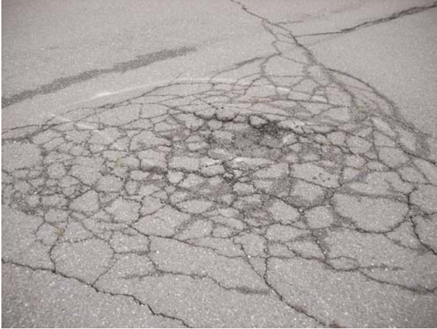
FIGURE 13 Pavement deterioration. Source: Lammerding 2010a.
