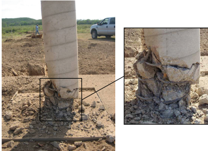
FIGURE 1 Observed direct shear failure state of column specimen (9).
