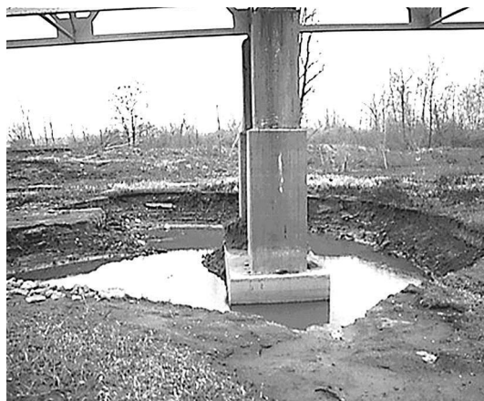
Local sediment scour at a bridge pier in a flood plain after a flow event.
