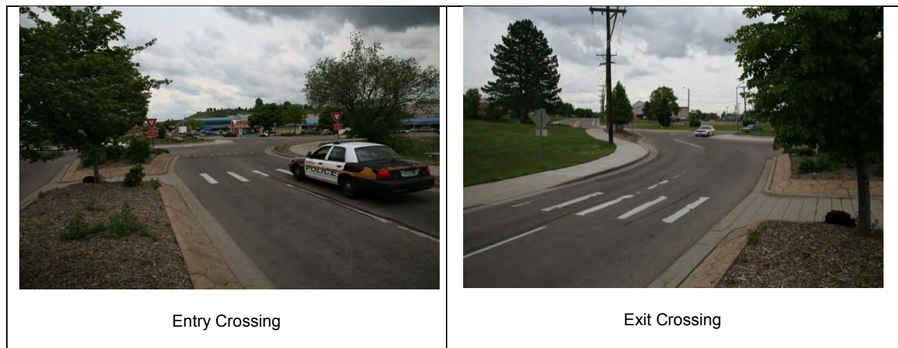
Exhibit 7 – HAWK signal test site prior to installation
