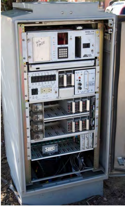
Exhibit 11 – 170 cabinet at test site in Golden, Colorado
