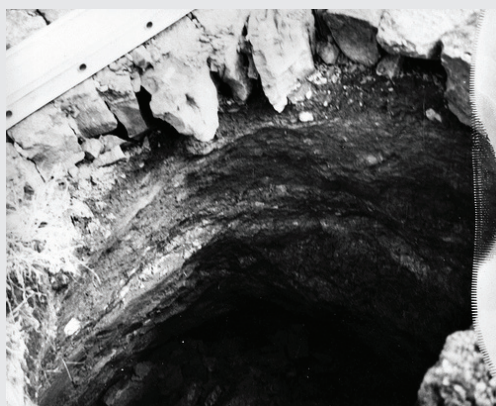
FIGURE 2 One of two sinkholes that appeared in the embankment of Wolf Creek Dam in 1968. SOURCE: USACE, Nashville District, 2011.
