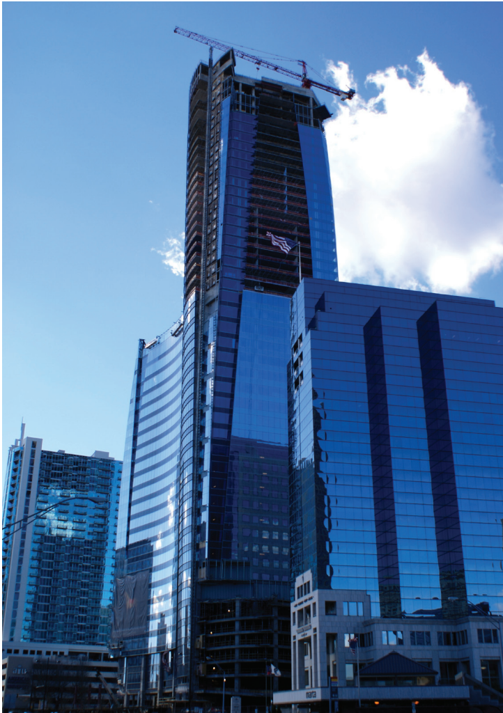
FIGURE 6 Construction of the Sovereign, Atlanta, Georgia. The building community uses climate information to make decisions about building materials, siting, and building design. These types of infrastructure decisions can have implications for decades. As the climate changes, information from climate models is being used as a guide to future climate conditions. SOURCE: Conor Carey, http://commons.wikimedia.org/wiki/File:Sovereign-Atlanta.jpg (accessed June 6, 2012).
