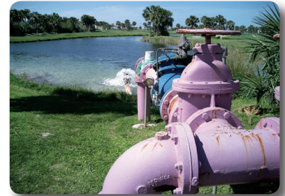
In the United States and other countries, purple pipes are used to distinguish nonpotable distribution systems, helping to prevent cross-connections.
