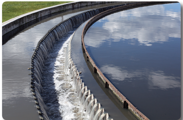
Secondary sedimentation basin in a wastewater treatment plant.
