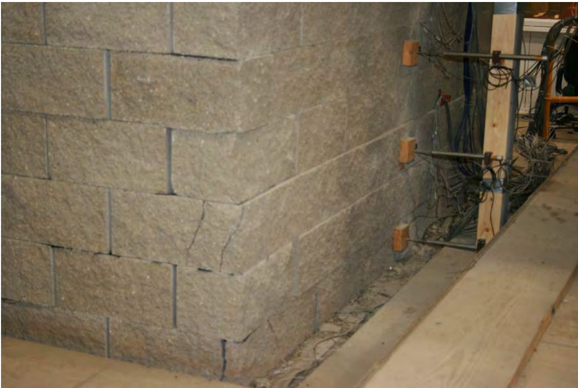
Figure 6.6: Photograph of Block Cracking after 0.67 g Test at 3 Hz
