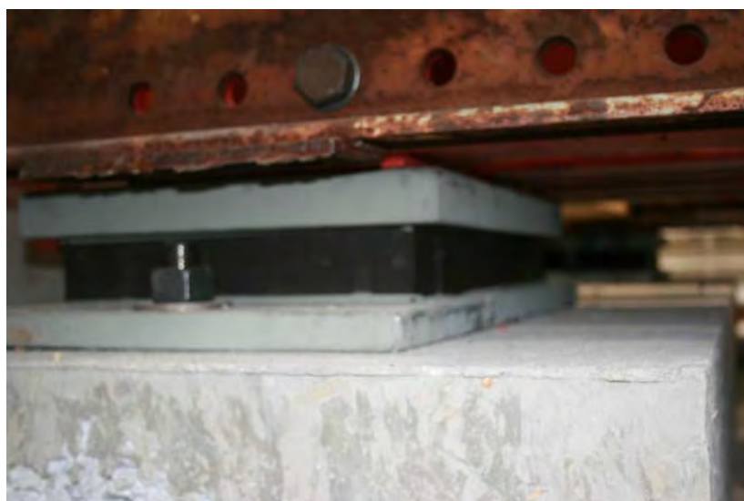
Figure 5.8: Elastomeric Pad Close-up
