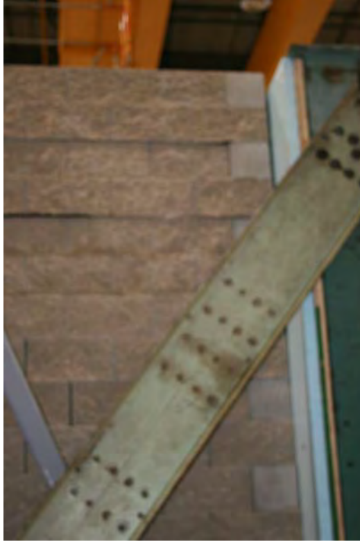
Figure 6.5: Photograph of Abutment Separation from Backwall after 0.15 g Test at 1.5 Hz
