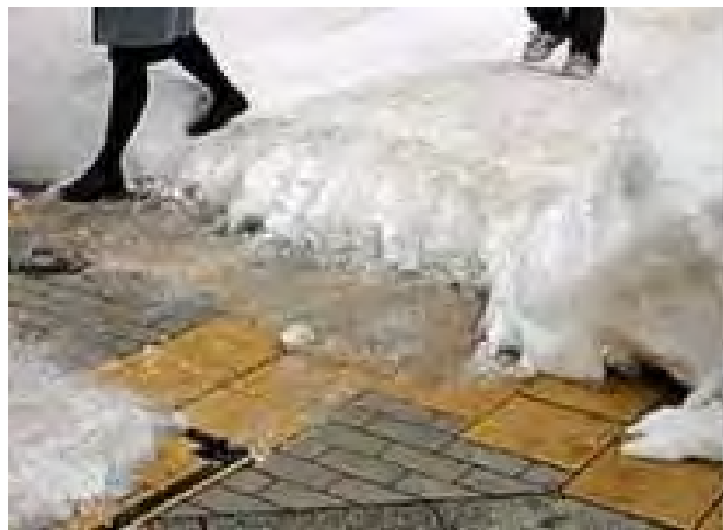
FIGURE 4 Example of poorly maintained sidewalk.
