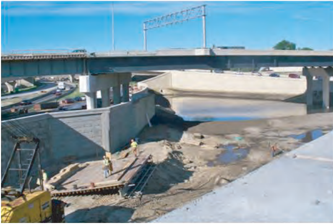
Figure 10.24. MnDOT I-35 retrofit, construction of the west commons pond, located beneath an elevated highway section.
