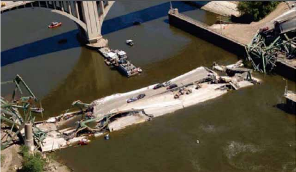
FIGURE 7 I-35W collapsed bridge section.
