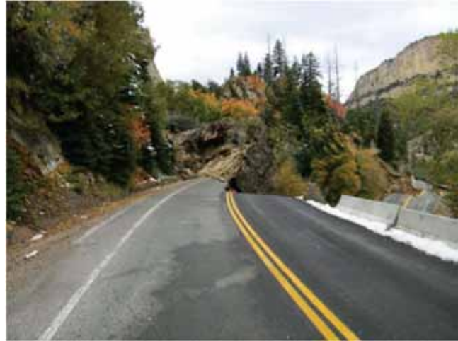
FIGURE 18 Aftermath of landslide on SR-14 (UDOT 2012).
