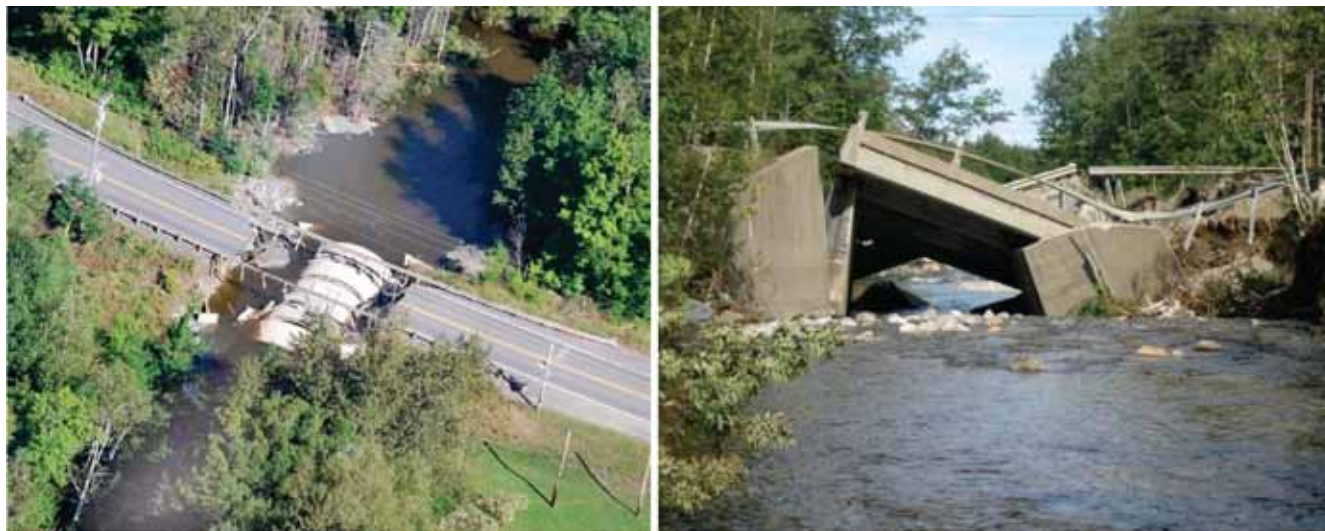
FIGURE 6 Damaged Route 27 Brackett Brook and North Branch bridges (Pulver 2012).
