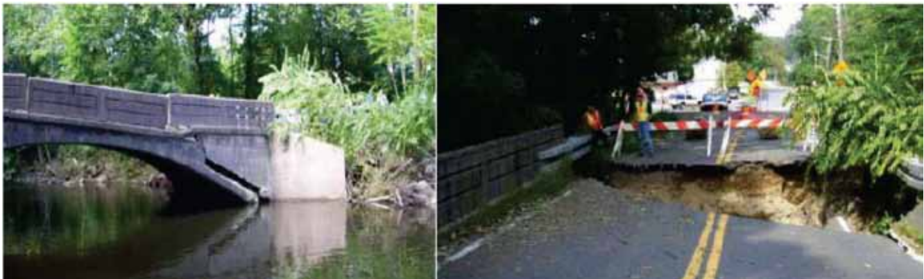
FIGURE 15 Ramapo River Bridge damage.
