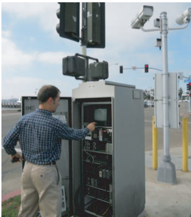
Figure H-20. Jon Hannasch conducts a system check on a red light camera system.
