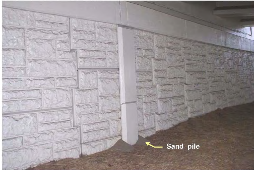
Photo 2. Pile of sand at base of slip joint
