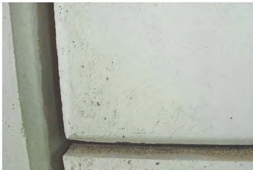
Photo 4. Sand in horizontal joint
