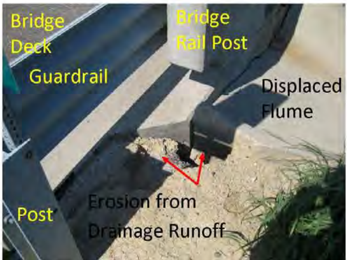
Improper drainage runoff from the roadway caused undermining of this road and displacement of the flume .
