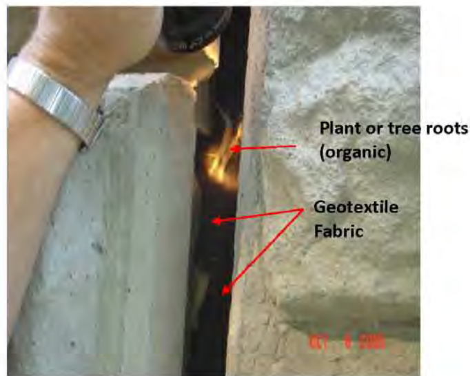
Organic material exposed outside of filter fabric (behind the wall face).
