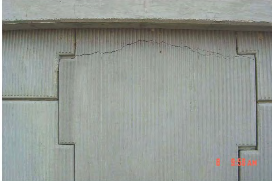
Photo 9. Crack in the facing panel
