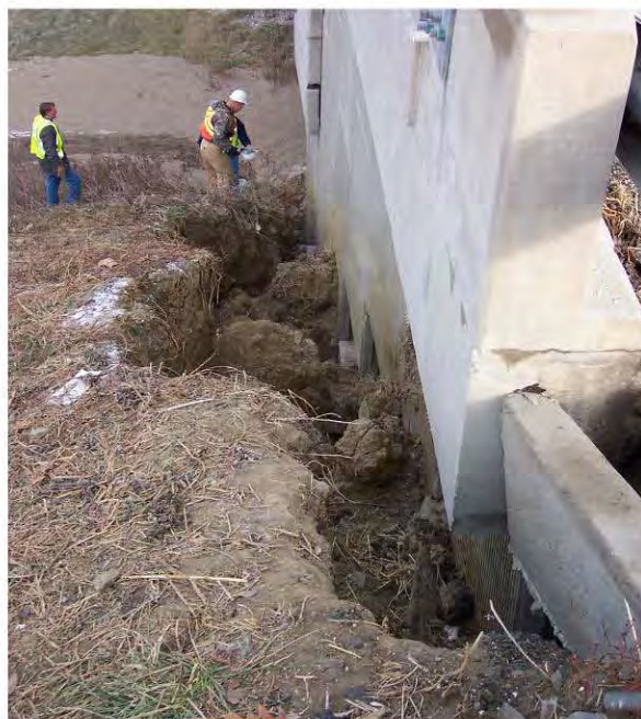
Photo 12. Severe erosion along the wall
