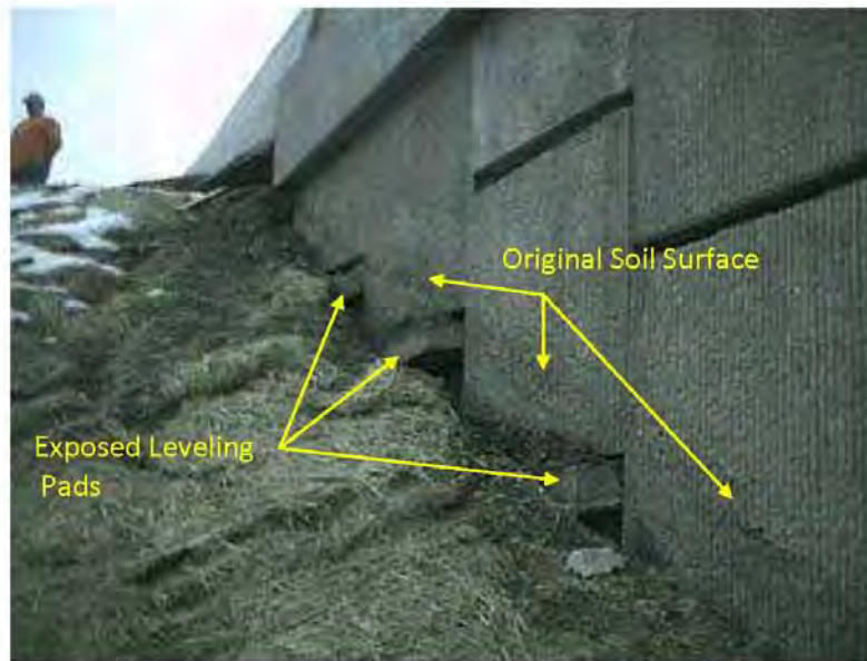
The soil surface along this wall is being eroded, which exposed the leveling pads.
