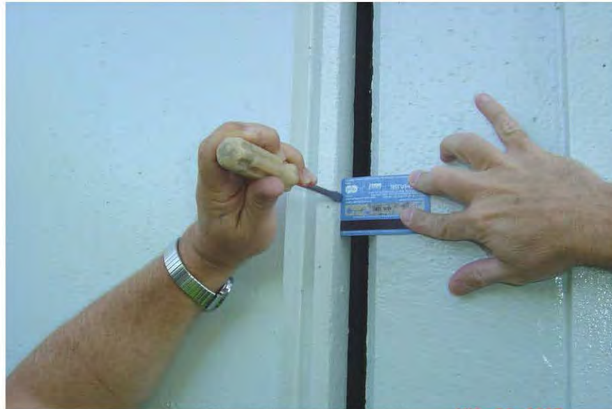
Photo 7. Panels offset at the joint
