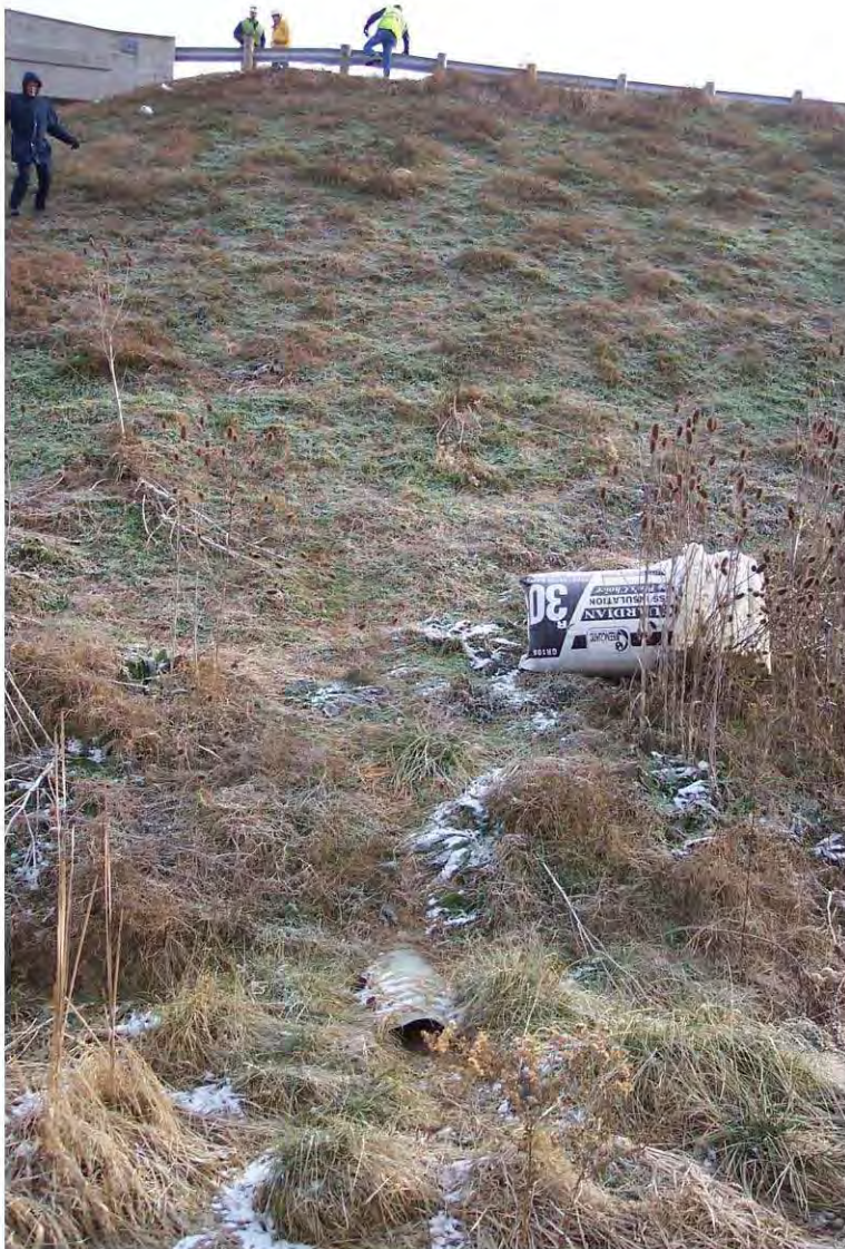
Photo 14. Blocked catch basin outlet
