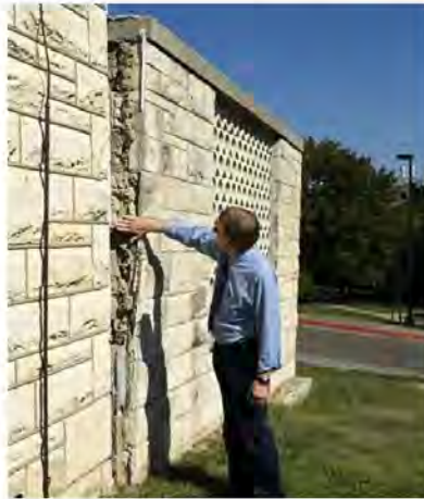
A panel wall showing a positive tilt.
