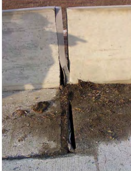
Photo 15. Large gaps at the approach slab
