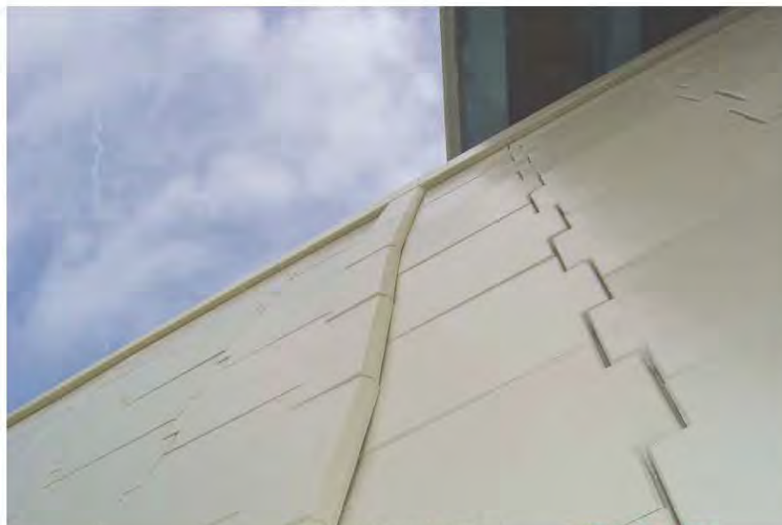
Photo 11. Bowed wall face
