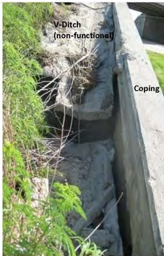
Loss of backfill has caused a complete break in this V-Ditch as well as its separation from the wall.
