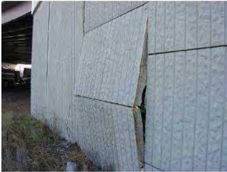
Bowing caused by failure of adjacent reinforcement connections.
