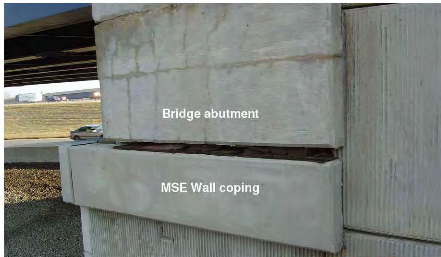
Photo 16. Opened joint between coping and abutment
