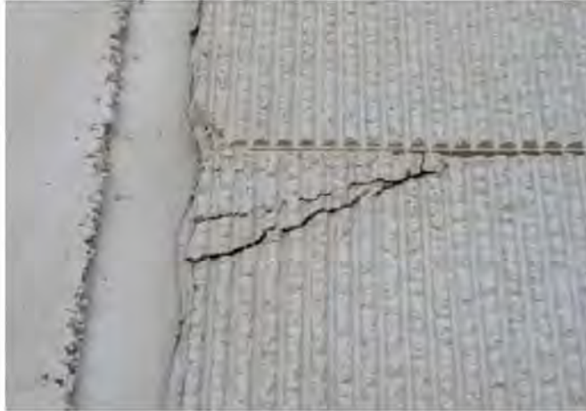
Separation of the corner on precast panel as a result of structural cracking.
