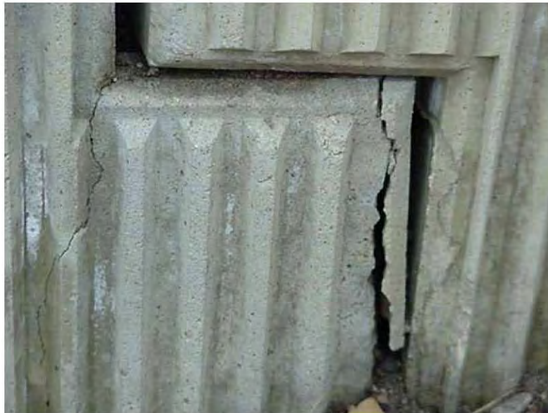
Photo 10. Cracks in the facing panel
