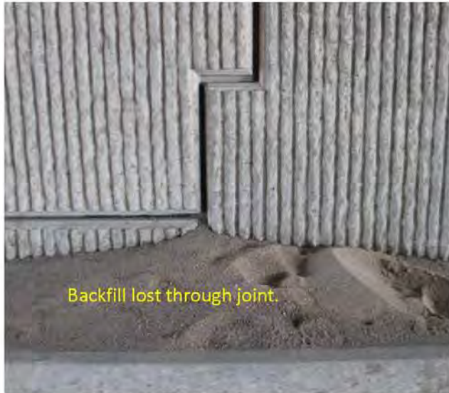
Loss of select backfill through joints.
