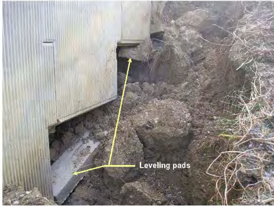
Photo 13. Leveling pad has been exposed by erosion
