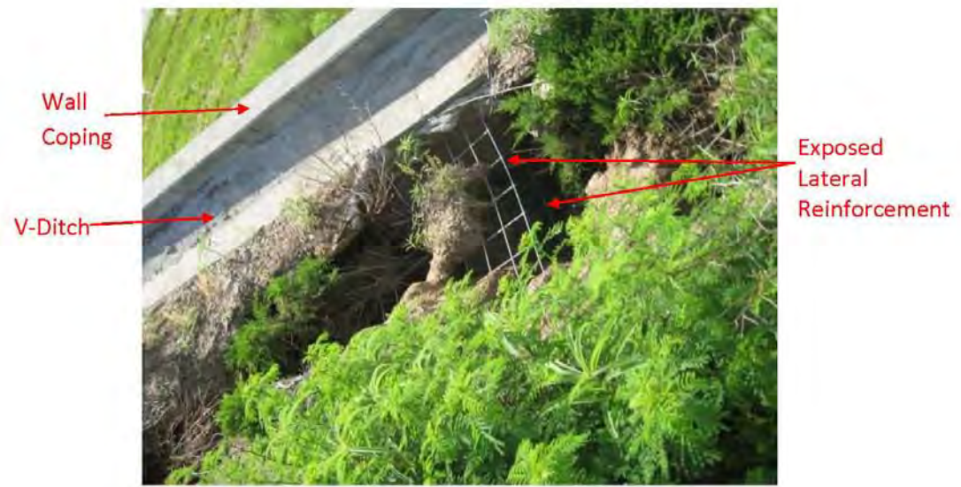
Washout (showing lateral reinforcement exposed).
