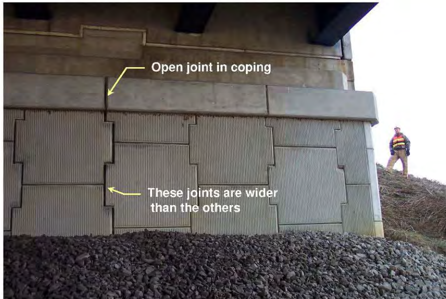
Photo 6. Nonuniform joint sizes and open joints in coping
