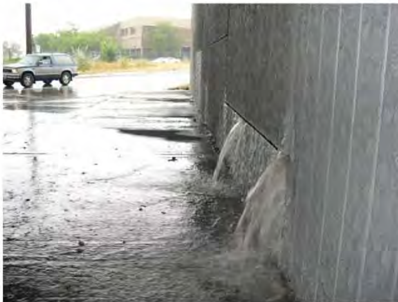
Problematic drainage is causing ponding at the front of this wall.
