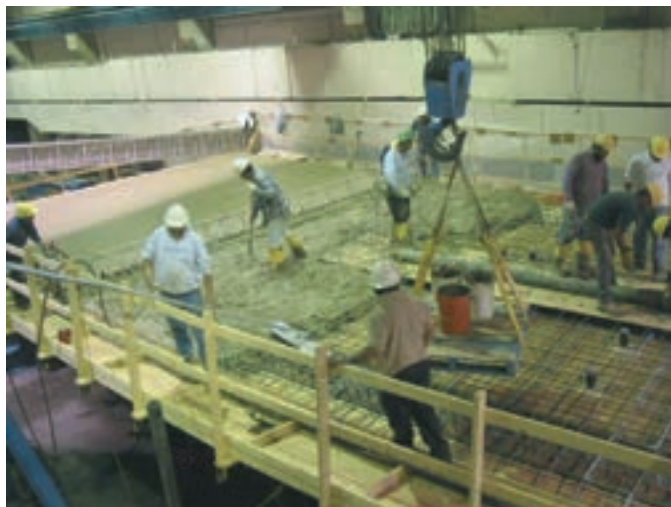
Figure 3-6. FHWA Test Bridge placement of the slab concrete (Jung, 2006; Jung and White, 2008).
