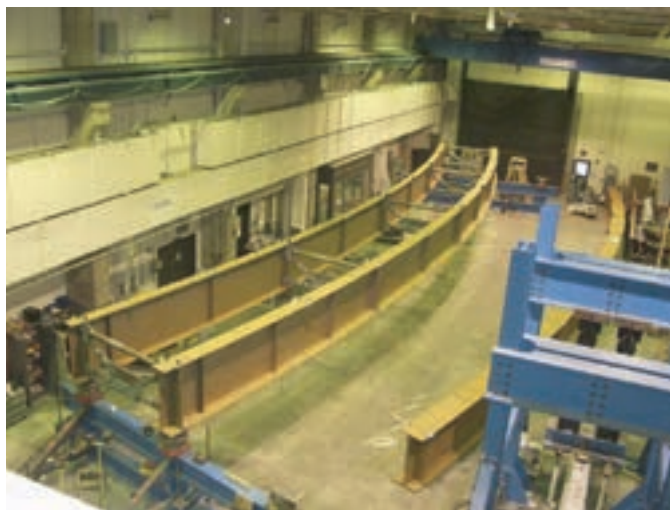
Figure 3-4. FHWA Test Bridge (EISCR1) during the steel erection, with cross-frames attached between girders G2 and G3 (Jung, 2006; Jung and White, 2008).
