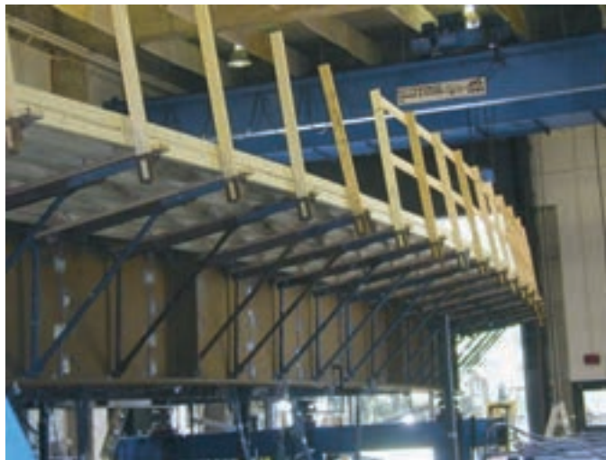
Figure 3-5. FHWA Test Bridge, overhang brackets attached to the fascia girder on the outside of the curve (Girder G1 per the NCHRP Project 12-79 naming convention, Girder G3 in reports and papers on the FHWA research) (Jung, 2006; Jung and White, 2008).
