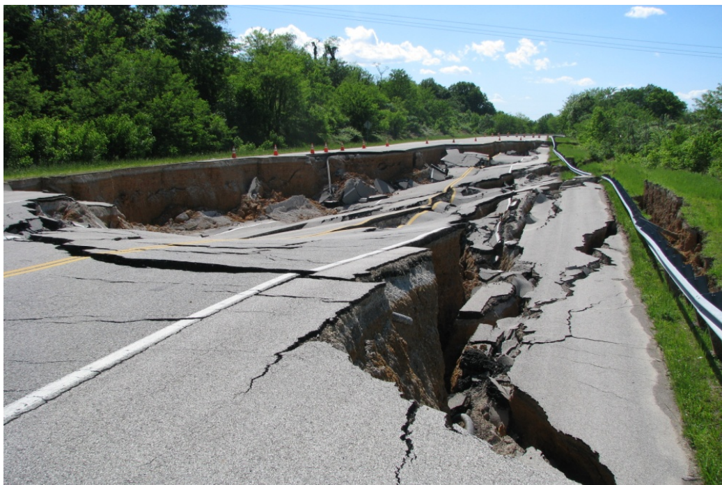
FIGURE 3 SR-7 in Maury County, Tennessee, after intense rainfall and record-level flooding in May 2010.
