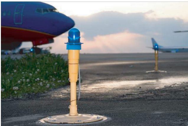
FIGURE 4 LED elevated taxiway edge light.
