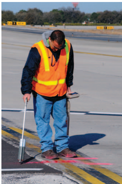
FIGURE 3 EML device in use to designate electric lines. (Photo courtesy of Cardno.)
