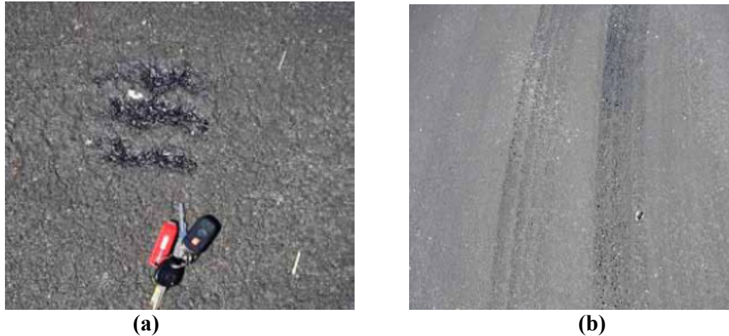
FIGURE 9 Double chip seal project problems at cul-de-sac locations: (a) excessive binder and soft spots in cul-de-sacs and (b) tearing of soft mat under turning traffic.
